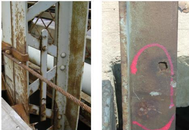
Figure 1. Typical corrosion observed in the steel structure of a low level bridge.
