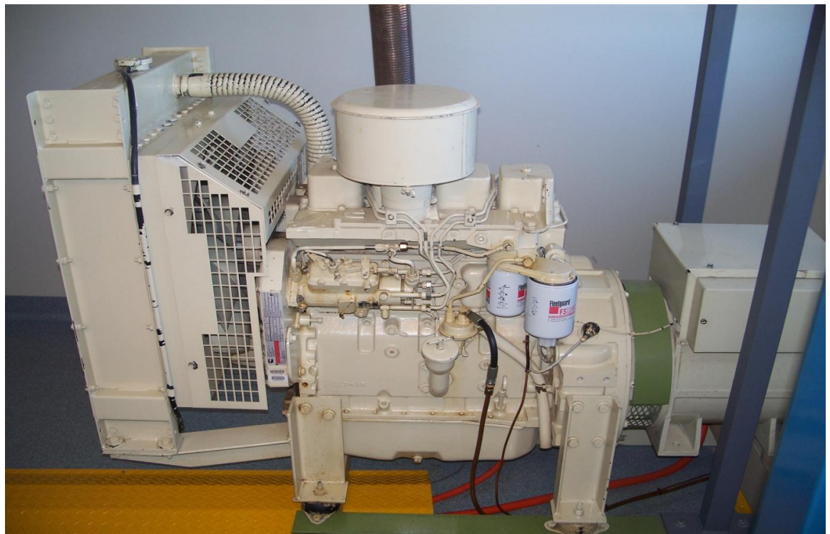
Figure 1.1: Diesel Backup Generator
