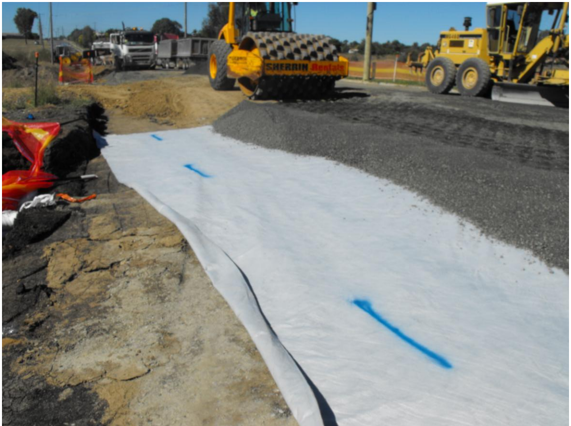
Figure 8.10 Placement of a geofabric on the clay subgrade to provide a working platform
