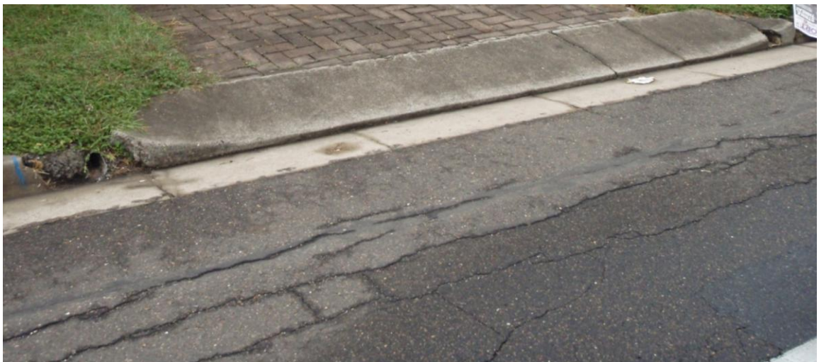
Figure 5.5 Longitudinal cracking and rutting on Whitehill Road, Raceview
