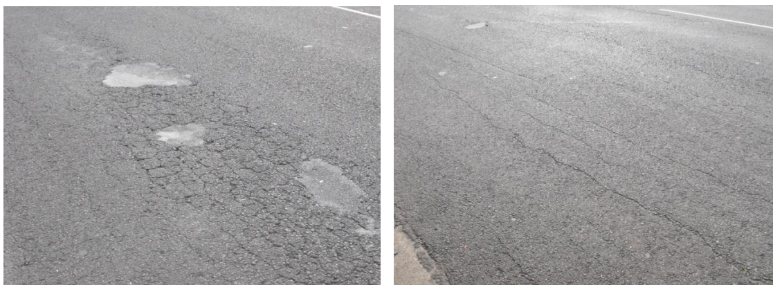
Figures 5.6 & 5.7 Robertson Road pavement failures
