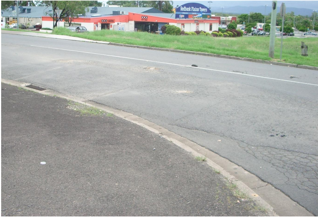
Figure 5.4 Severe crocodile cracking and rutting on Redbank Plains Rd, Redbank Plains
