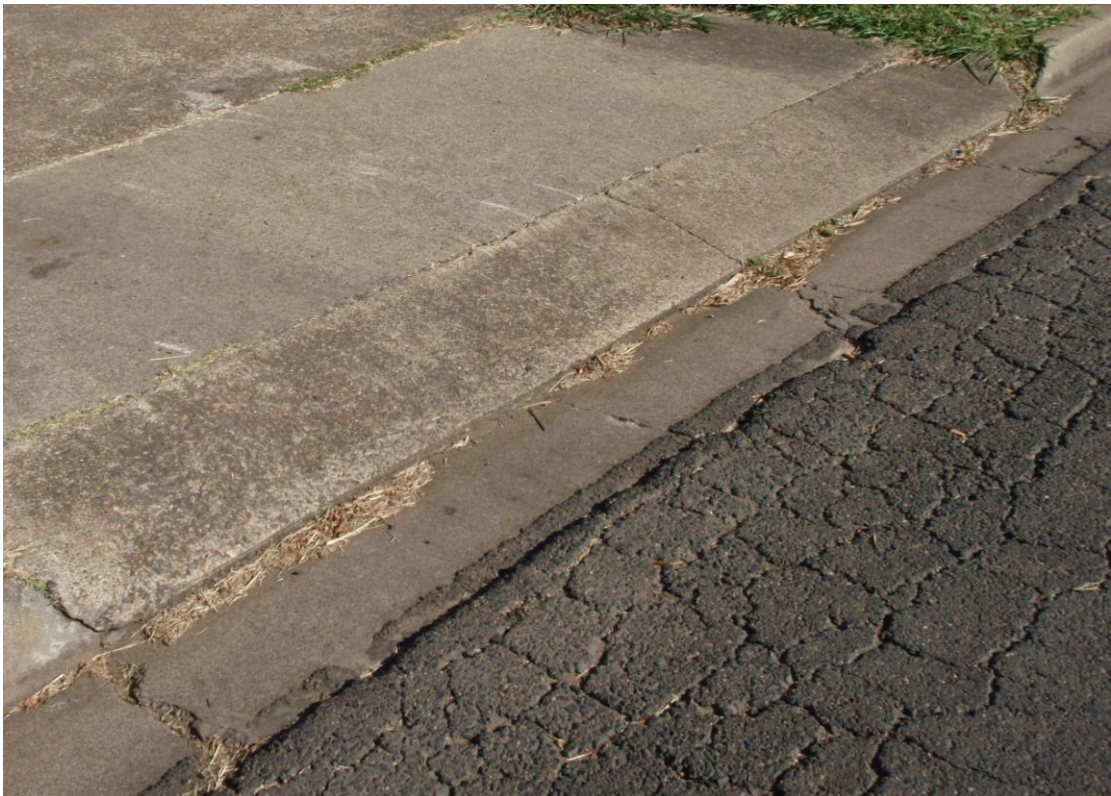
Figure 5.8 Crocodile cracking and kerb and channel deformation on South Station Rd
