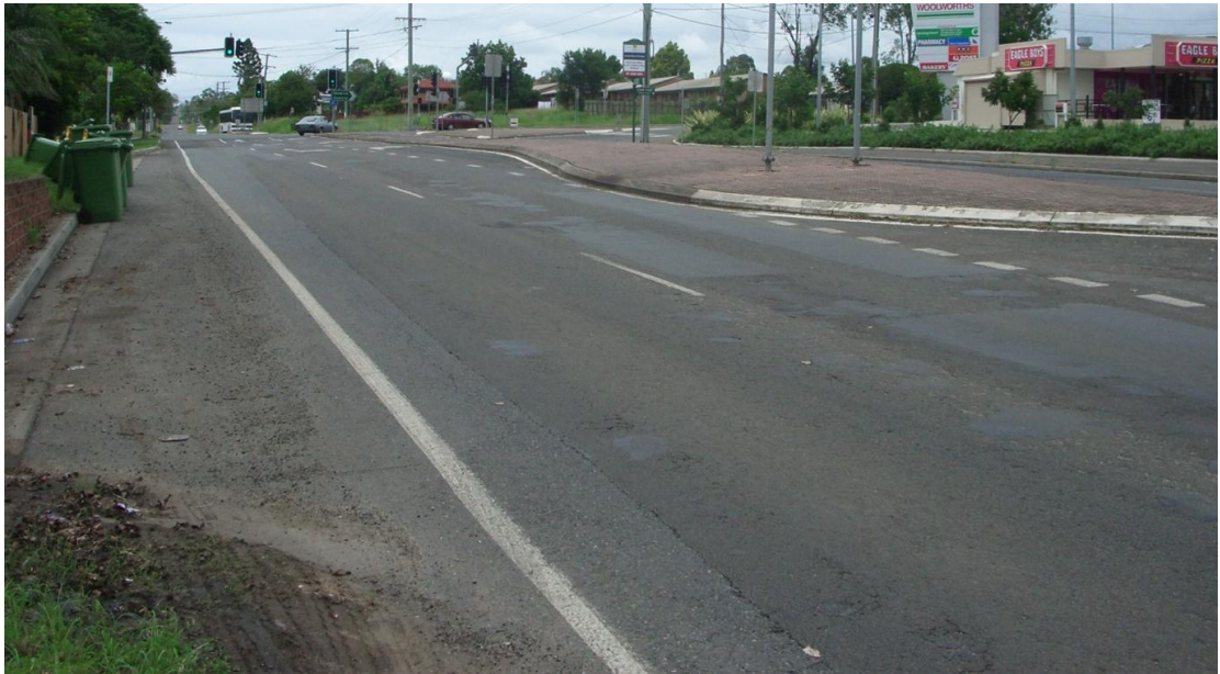
Figure 5.3 Pavement failures at Redbank Plains Rd, Redbank Plains
