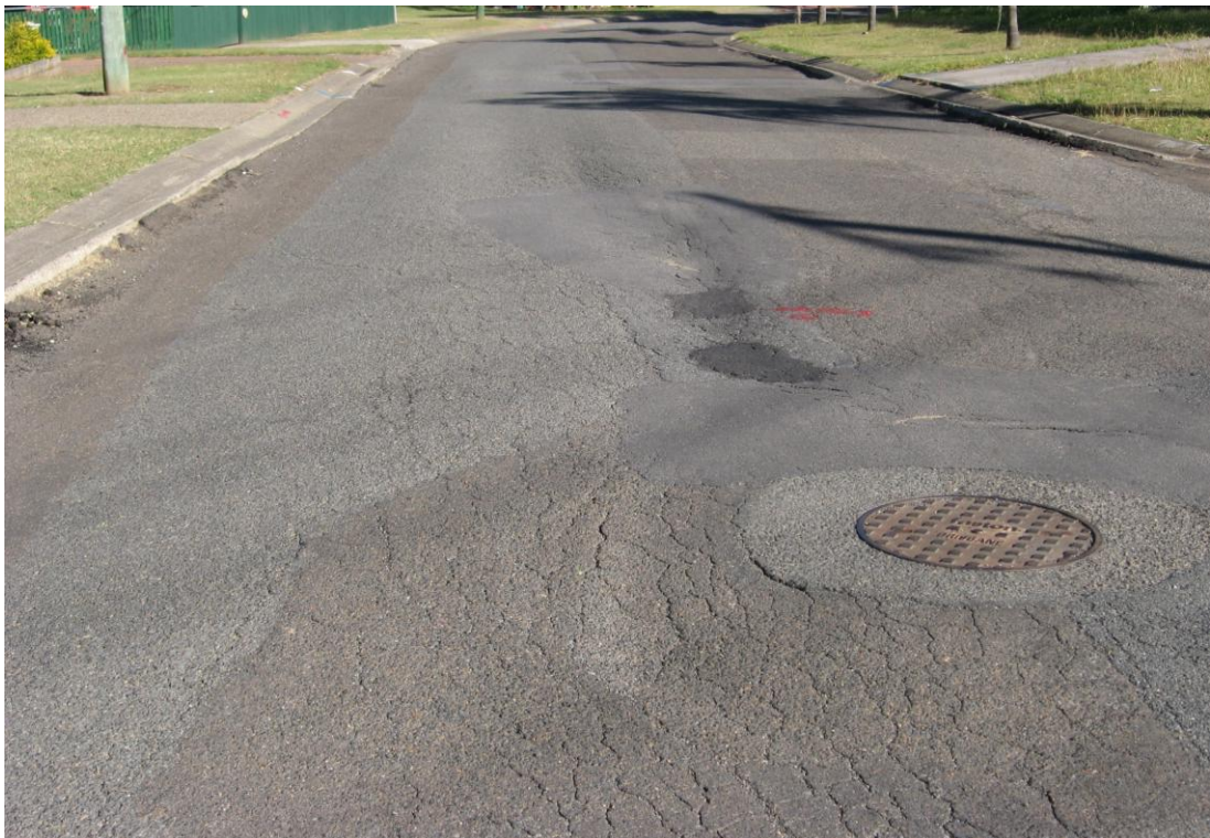
Figure 5.9 Josey Rd pavement condition
