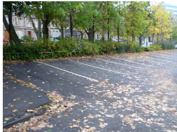
Fig. 3. The existing carpark showing cracks and de-gradation due to existence of foundations
