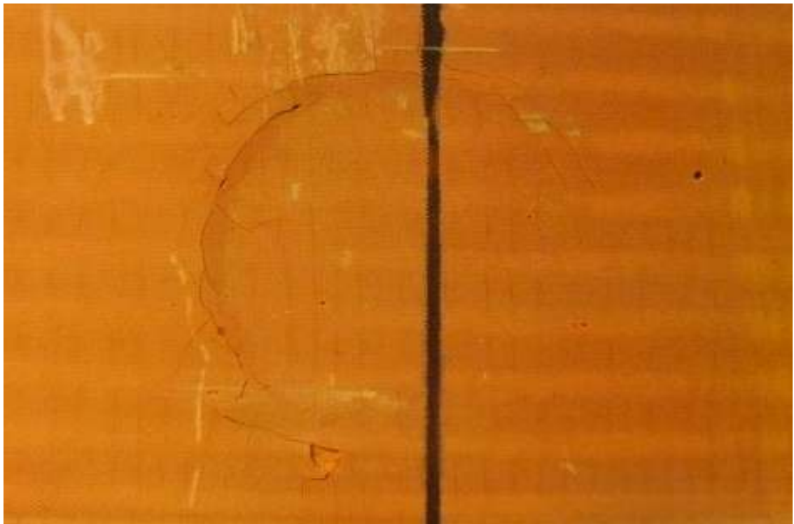
Figure 4.2 Blunt Impact Damage
