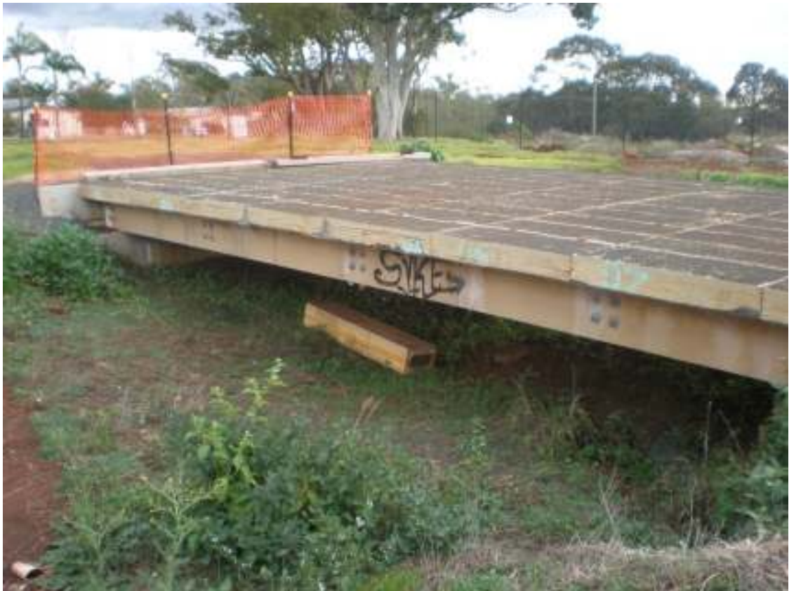
Figure 1.1 Vandalism on fibre composite bridge
