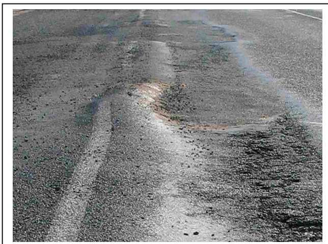
Figure 2-6 - Shoving in Road Surface
