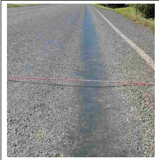
Figure 2-5 - Rutting in Road Surface
