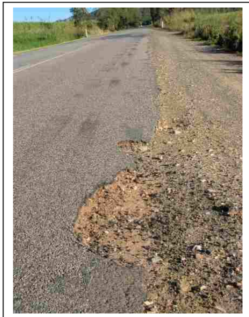
Figure 2-12 - Edge Failure along Road
