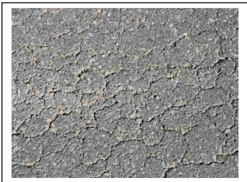
Figure 2-10 - Crocodile Cracks in Road Surface
