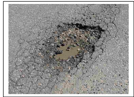
Figure 2-11 - Pothole in Road
