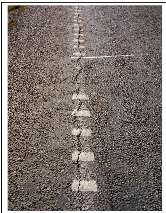
(a) Longitudinal Crack at edge line
