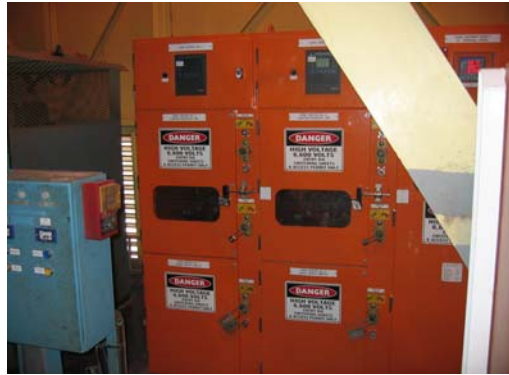
Fig. 5.1 VCB cabinet with warning signage
