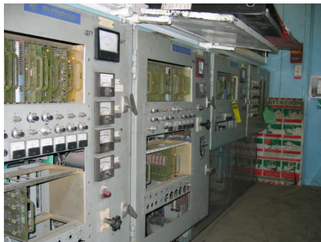
Fig. 5.6 Power Control Room – Note the racks of vertical electronic cards
