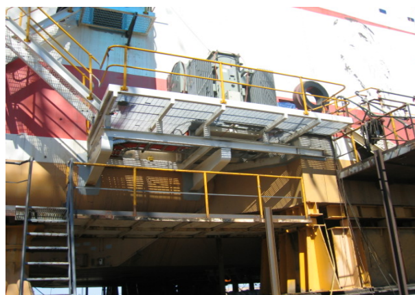
Fig. 5.2 Air cooled transformer mounted external to revolving frame
