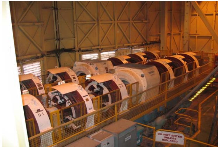
Fig. 5.3 DC Generator banks
