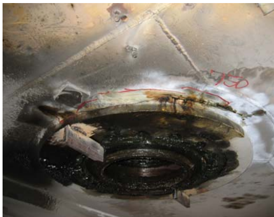
Fig. 6.2a Fabricated section in situ showing cracks
