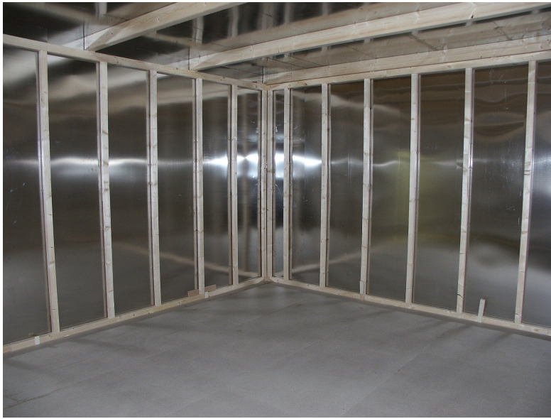
Figure 1.5.: Final stage of construction of the inner shielded room. View towards the N-E corner. Mu-metal is in place but not yet covered with plasterboard.
