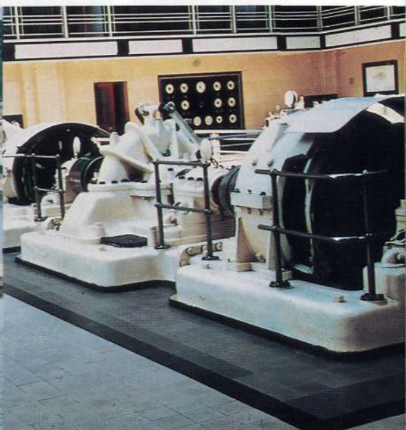
3.3 Interior of a pumping station of the Thames Water Authority.
