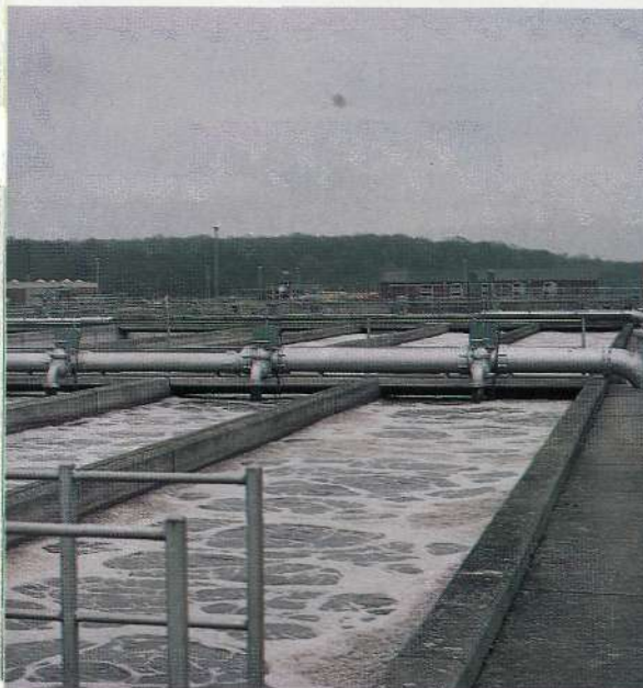
4.2 Basingstoke sewage works: activated sludge tanks.
