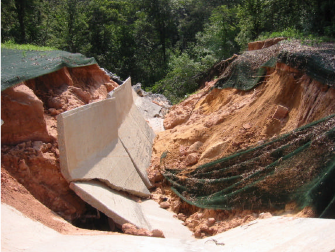
Figure 15. Stormwater drainage failure in Liberty County, Florida.
