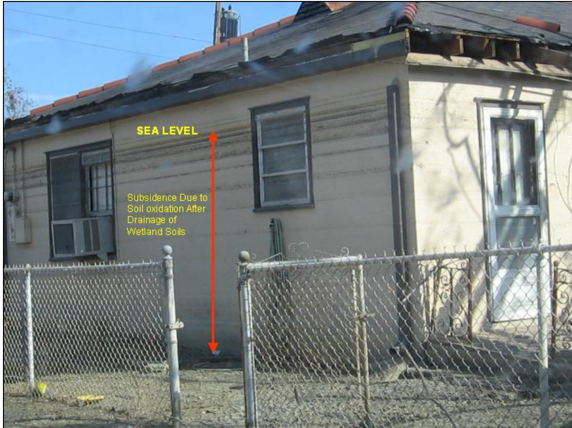
Figure 7: A house in a lower section of New Orleans that was flooded to nearly the roof, as shown by the series of water marks. Note the door height is a standard six ft six inches and thus the level of water was from the ground nearly 8 feet deep. The level of land subsidence is shown by the red arrow and indicates that the soil had a subsidence of nearly 6 + feet due to drainage of the wetland soils and compaction by dense building on soils of low bulk density.
