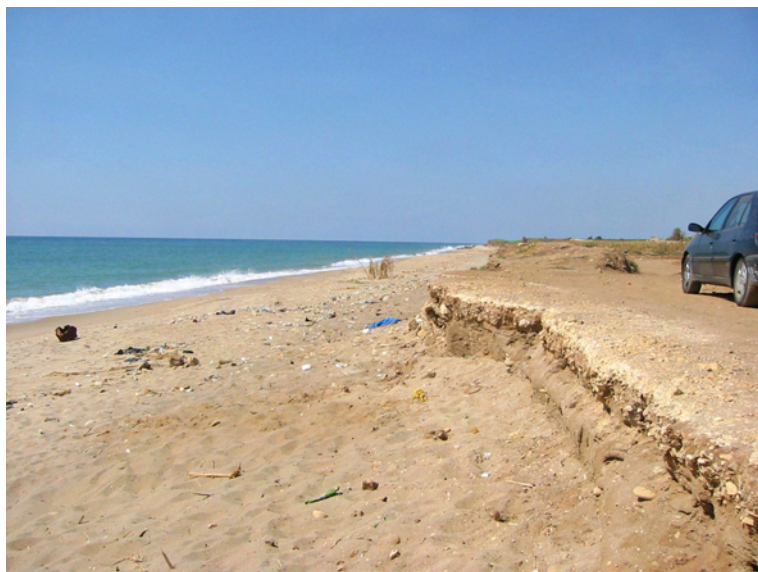
Photo 17: Beach erosion and subsidence
