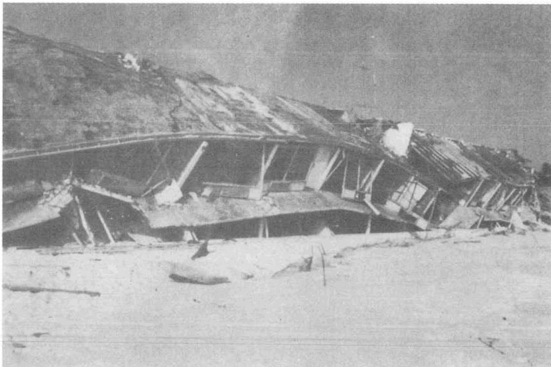
Figure 16c. Hurricane Juan (1985) damage (From Clark, 1986a).
