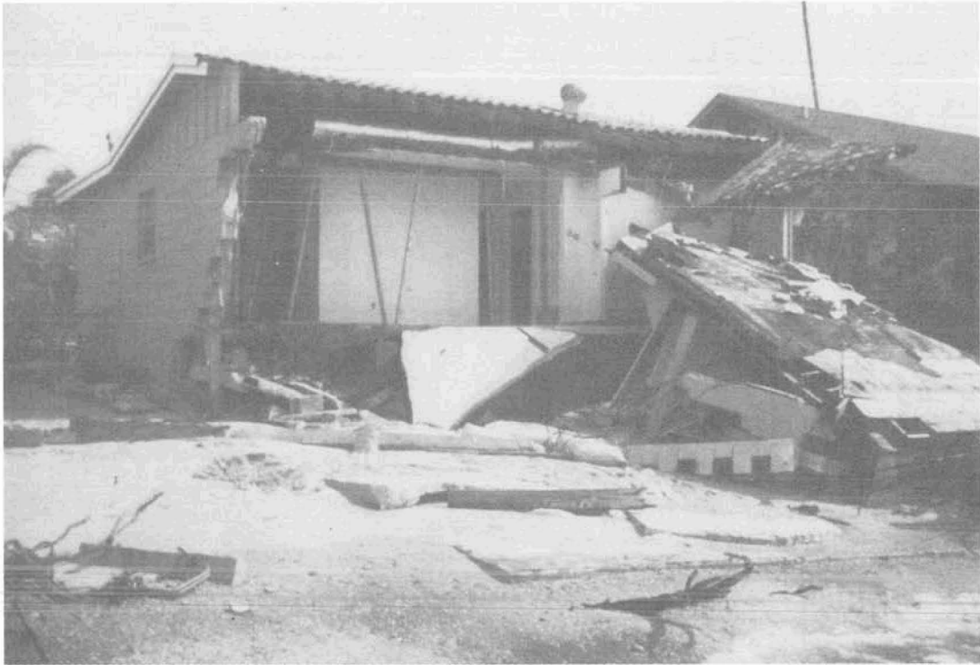
Figure 16a. Hurricane Juan (1985) damage (From Clark, 1986a).
