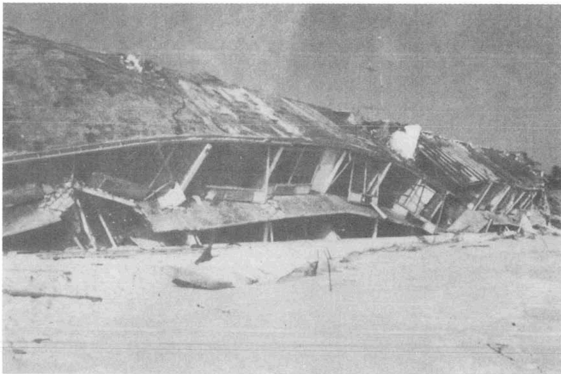
Figure 16c. Hurricane Juan (1985) damage (From Clark, 1986a).
