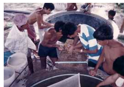
Fig. 7. (Bottom) Chinese circular hatchery being constructed by Mr Phoung Phun in Prey Veng district.
