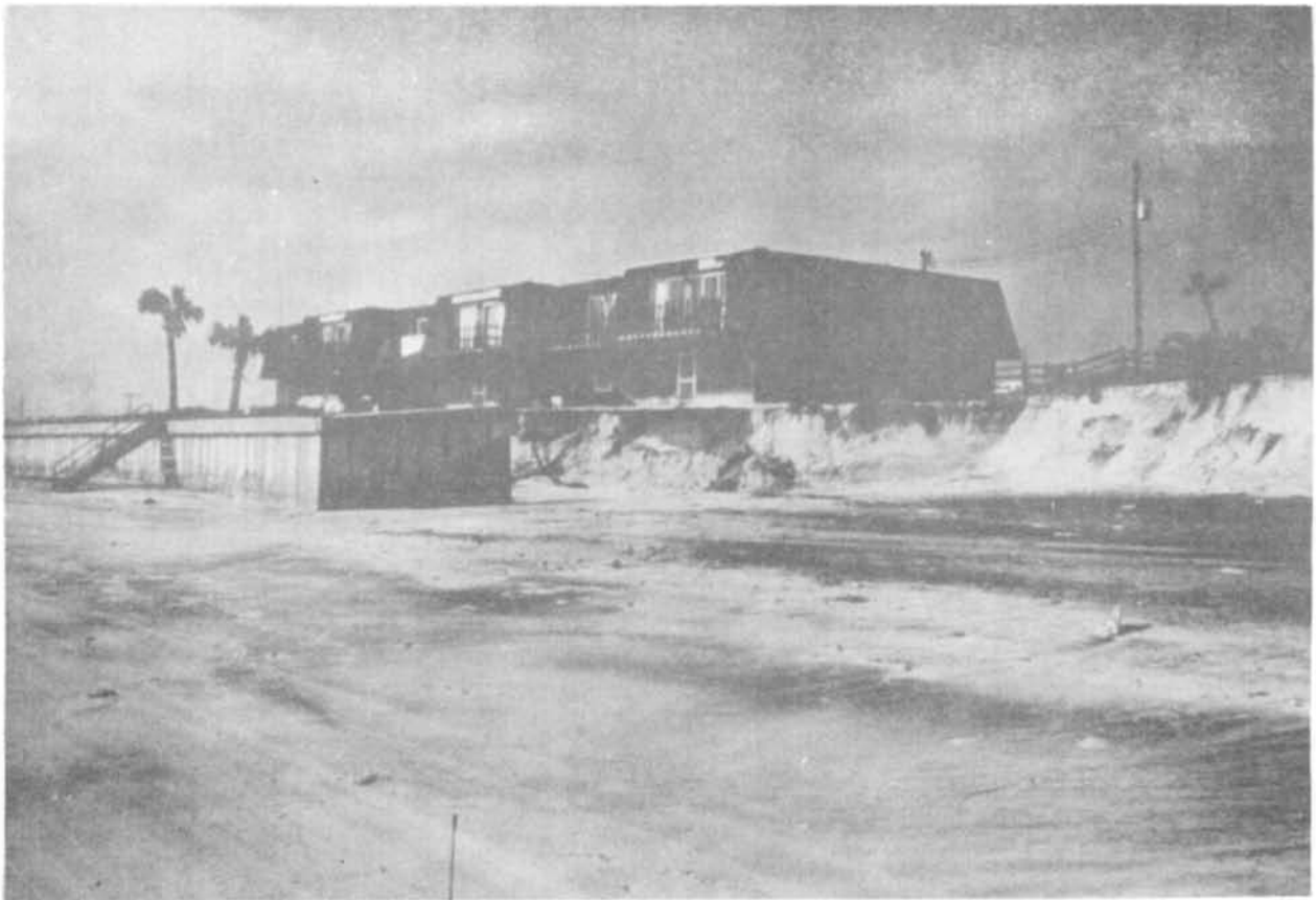
Figure 6. Inadequate Return Wall Length (Courtesy of Professor Byron Spangler)
