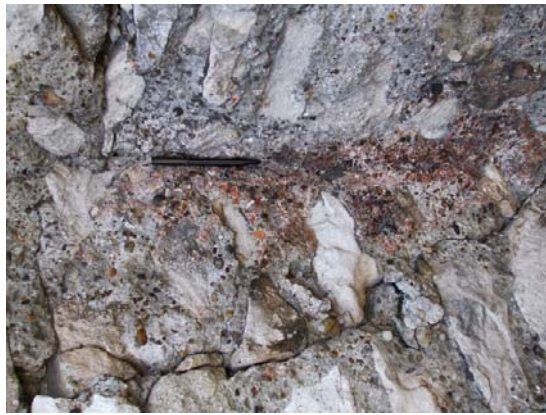
Fig.112 Detail showing the use of brick's fragments as aggregates in a repairing mortars. Aquincum.
