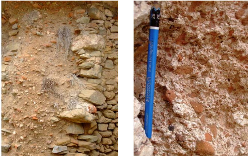
Fig.100-101 On the right a detail of wall in opus caementicium , on the right a detail of structural mortar with brick's fragments of different sizes ( cocciopesto ) (Galerius Palace in Thessaloniki)
