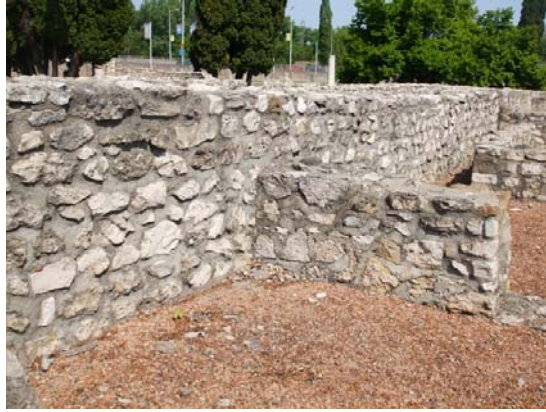
Fig.113 The large use of cement in the restoration of walls. Aquincum.
