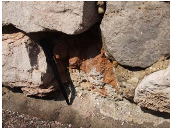
Fig.79 Detail of mortar during the sampling. Presence of brick as elements of the structure but not brick's fragments as aggregate in the mortar.
