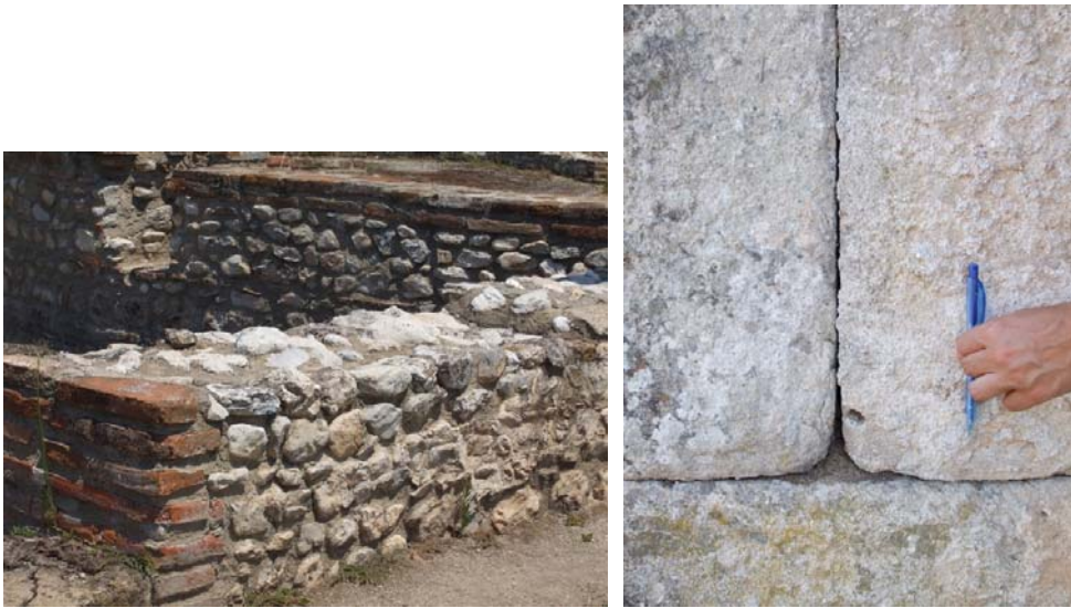
Fig.104 Detail of walls in opus mixtum , Fig.105 Detail of well shaped building stones constituting the wall without the use of any binder
