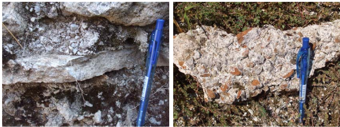
Fig.108-109 Details of different mortars: on the left a detail of structural mortar showing the absence of brick's fragments as aggregate, on the right a specimen of mortar used as support of mosaics, containing a large amount of brick's fragments of different sizes ( cocciopesto )
