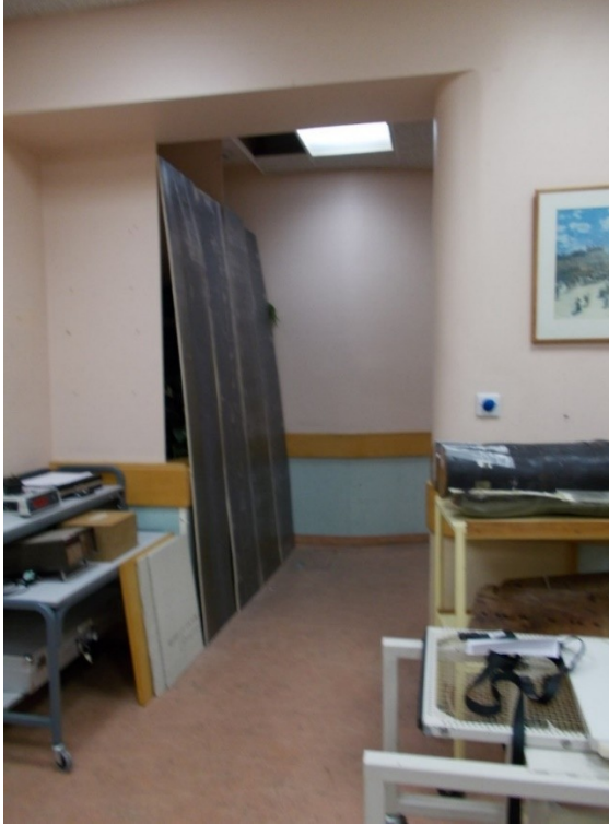
Figure 2. Treatment room view of the maze showing lead-lined plywood boards partly covering triangular section of maze wall.
