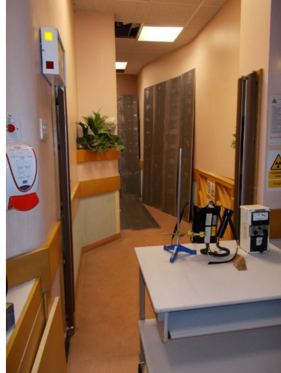
Figure 3. Maze entrance view showing lead-lined plywood boards partly covering Maze triangular section of maze wall, adjacent maze wall and floor. Two portable dose-rate meters are shown in position at the maze entrance.
