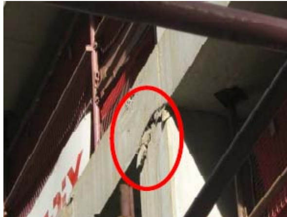
Figure 2: Defect in the column located at the fifth floor
