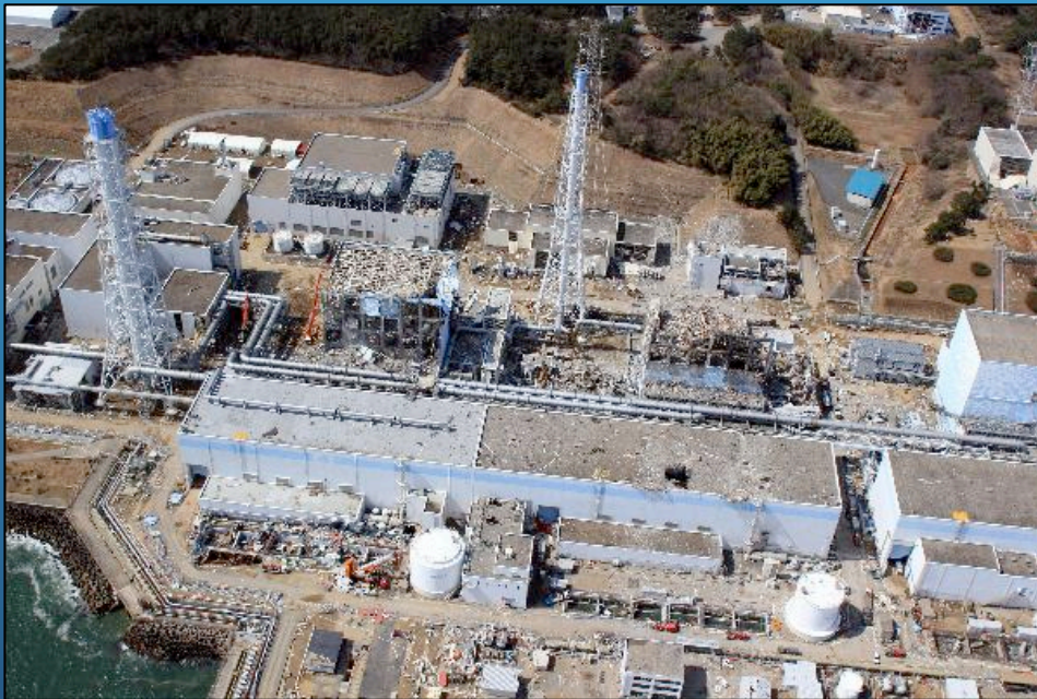
Damage to Fukushima Dai-ichi nuclear power plant - photo taken from a UAS. (AP Photo/Air Photo Service)
