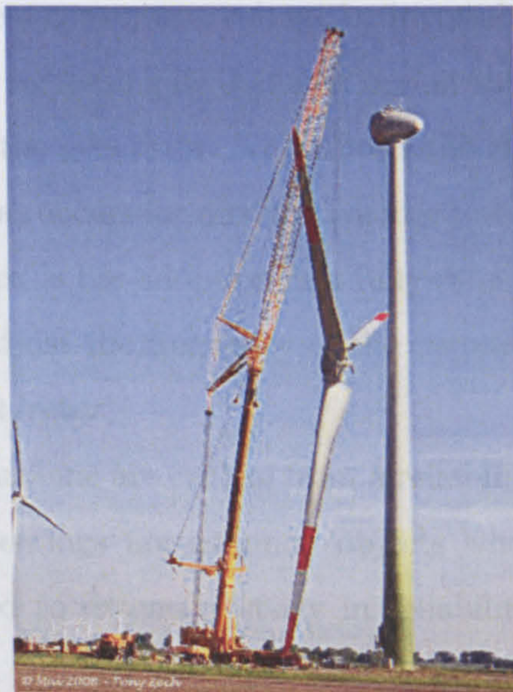
Figure 4.2: A rotor of a direct drive machine, being mounted on the nacelle [66]
