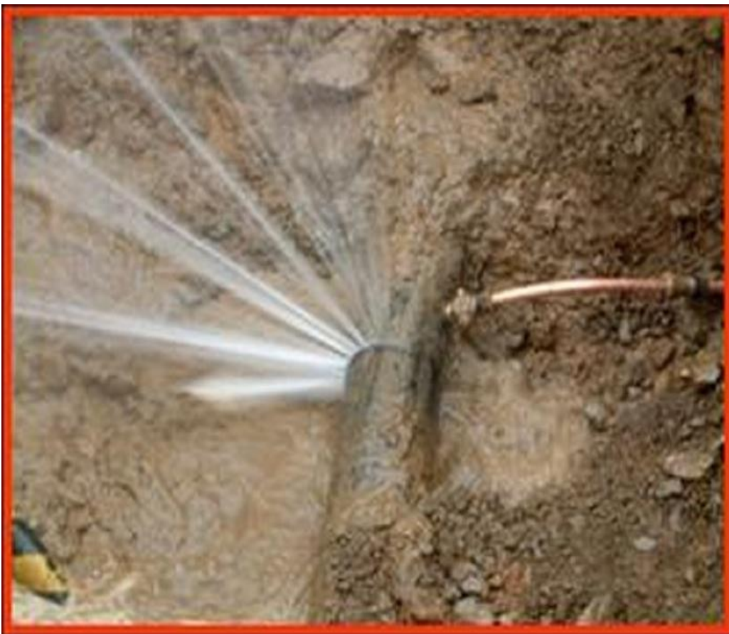
Figure 3-9 Leaks in pipe carrying water (KillickPlumbing, 2008)
