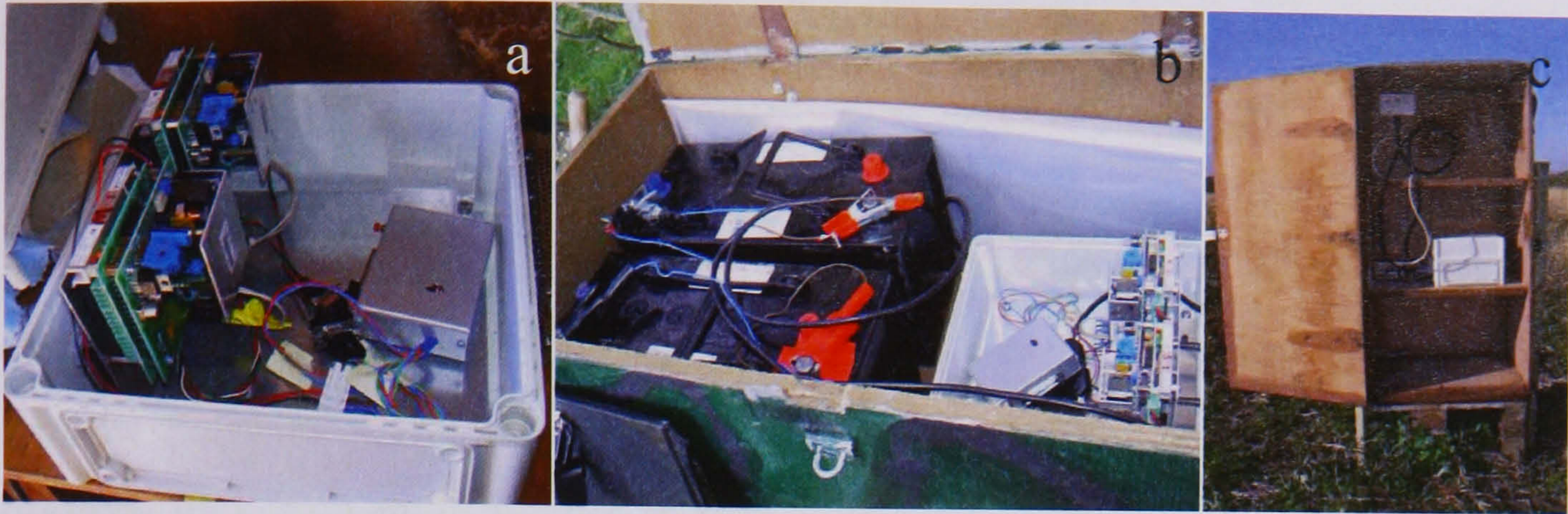
Figure 3.10 (a) Waterproof box with two units (master and slave), each containing a reader module and a control module, on the left and logger box on the right (b) Battery powered detector showing two 110Ah 12V batteries and reader/control box all housed in a protective wooden box (c) Wooden housing of PIT equipment for mains powered reader showing mains power supply, step-down transformer and reader/control box
