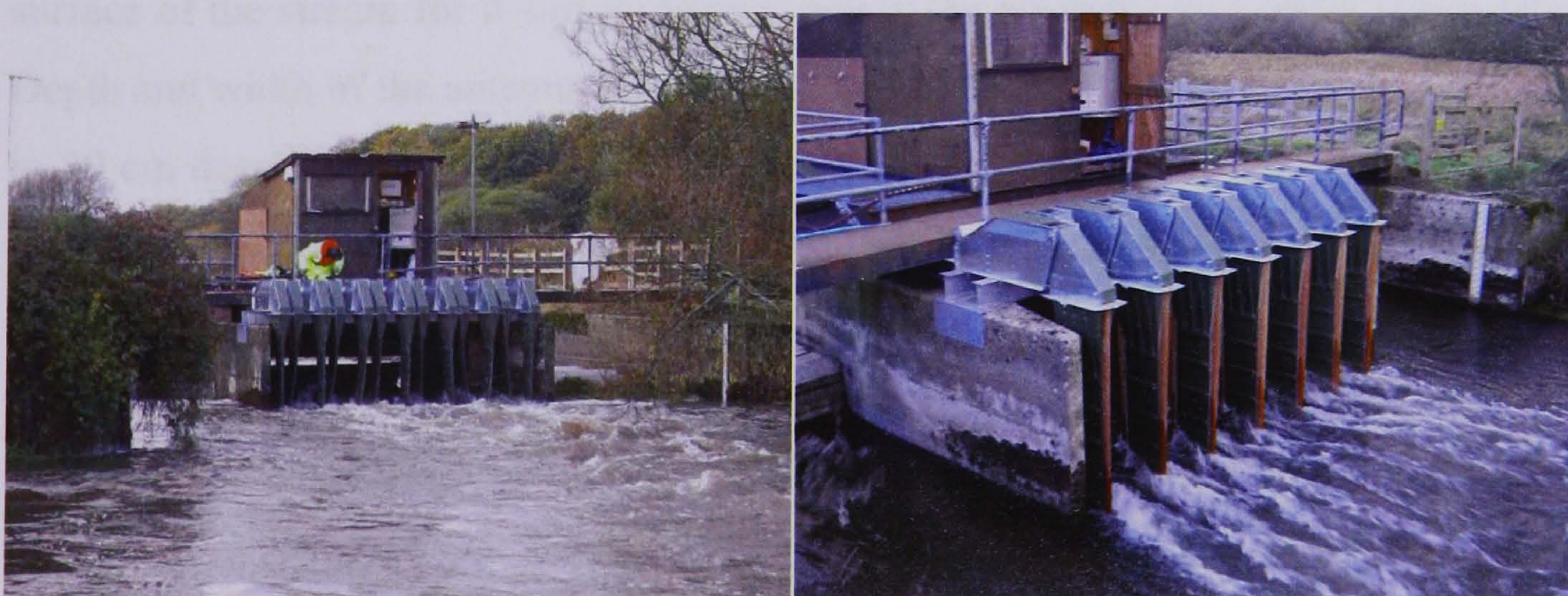
Figure 3.9 UKID PIT detector on the main River Frome at East Stoke, comprising 13 multiplexed antennae attached to hydraulic vanes. The vanes lift every four hours to clear any debris caught on them.
