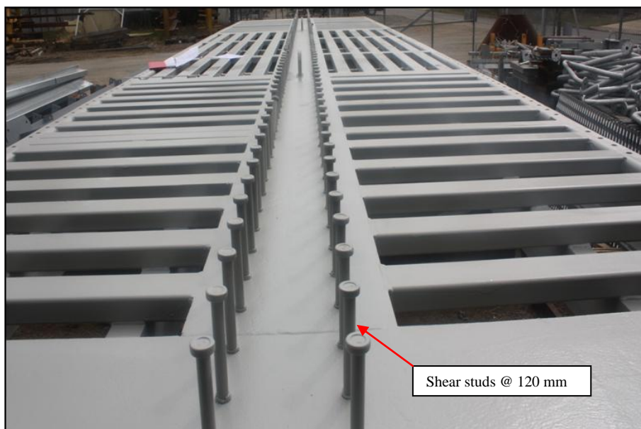
Figure 5.11 FRW ready for installation after sand blasting and corrosion paint applied; shear studs were welded on the main box girder in the fabrication yard
