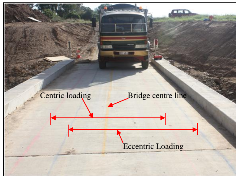
Figure 6.4 Test truck and markings on the slab to assist the driver to position the truck for different load tests
