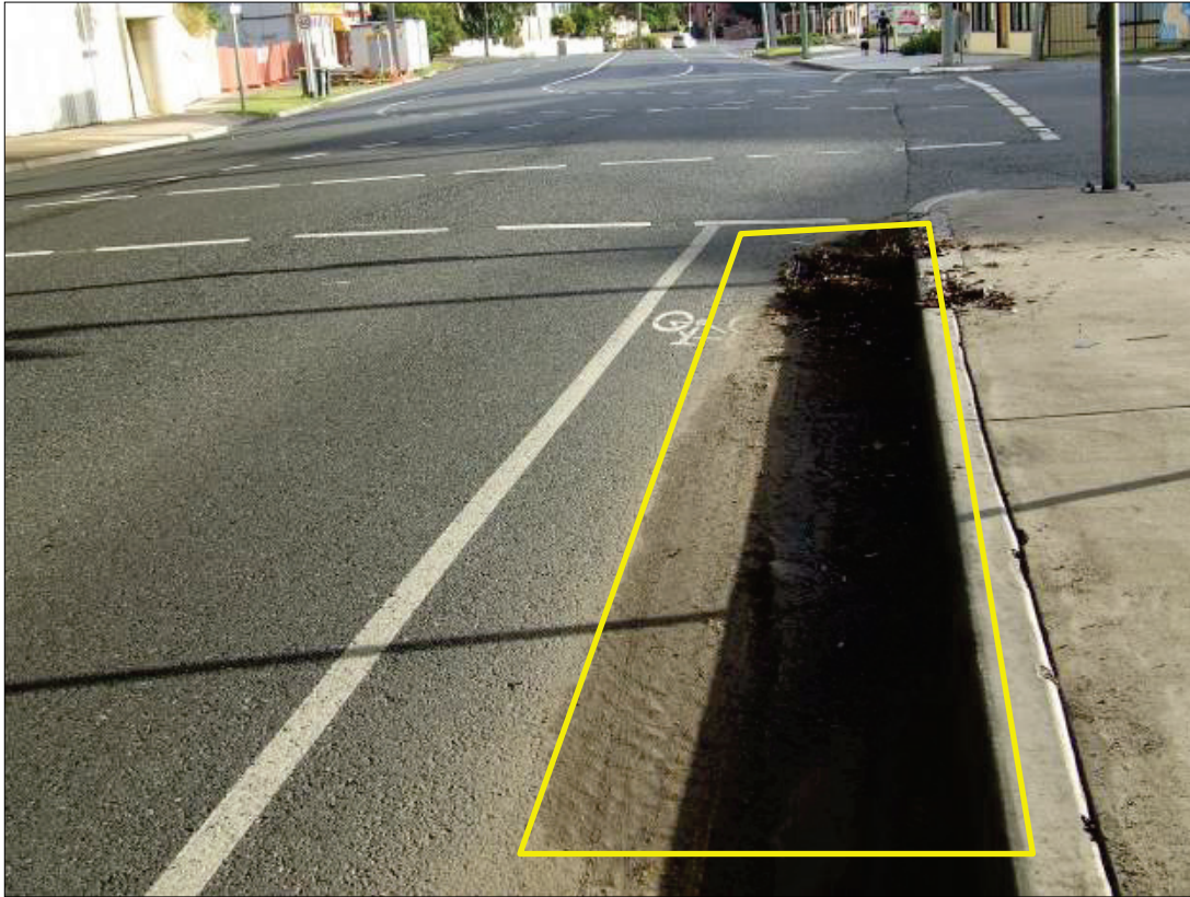
Figure 4.12 In the vicinity of stormwater drain (Figure 4.11) in fine sediment residue is an accumulation of traffic dust and organic material after a wet weather period (T junction between Park Road and Annerley Road, South Brisbane). This creates hazardous conditions for cyclists (May 2008).
