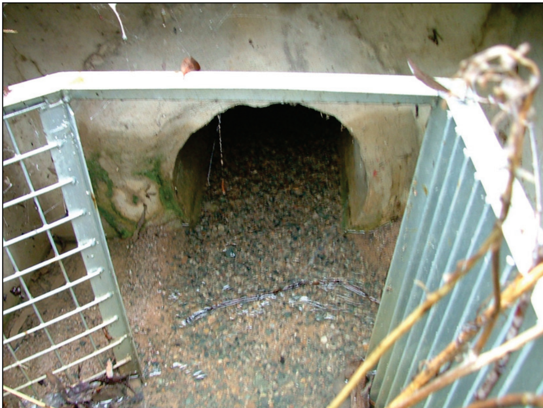
Figure 4.24 The view of the pipe inlet attached to the GPT in Figure 4.23. Fine sediments deposited are a result of a low incoming stormwater flow rate.
