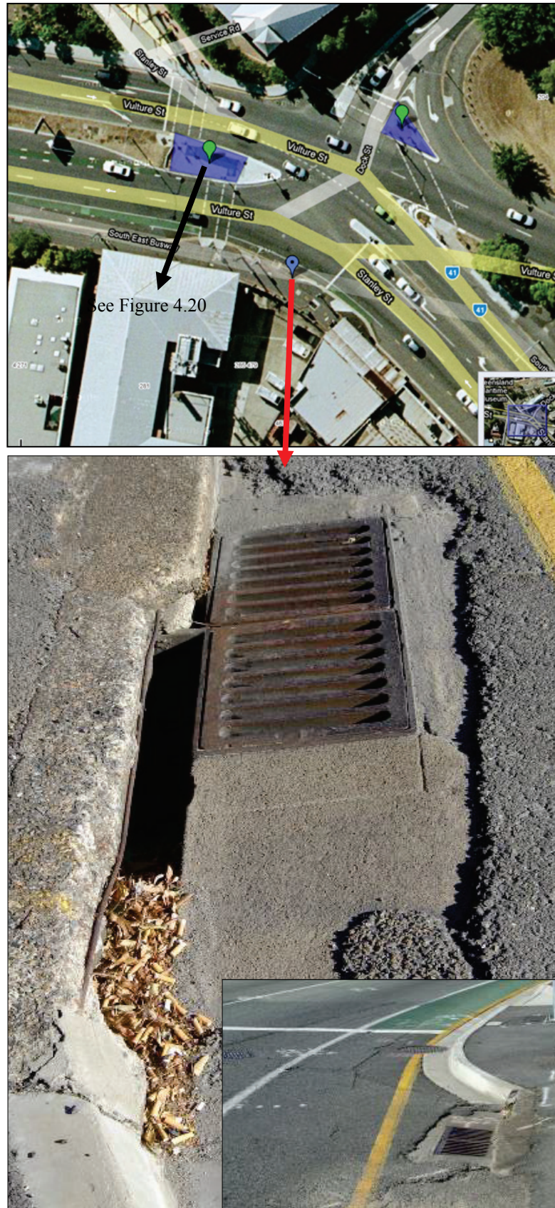
Figure 4.19 This drain is located on a pedestrian crossing at a busy intersection along the Brisbane River. The roadside gutters at the pedestrian crossing are commonly used to dispose of cigarette butts. Lower right shows the drain at the road intersection (October 2007).
