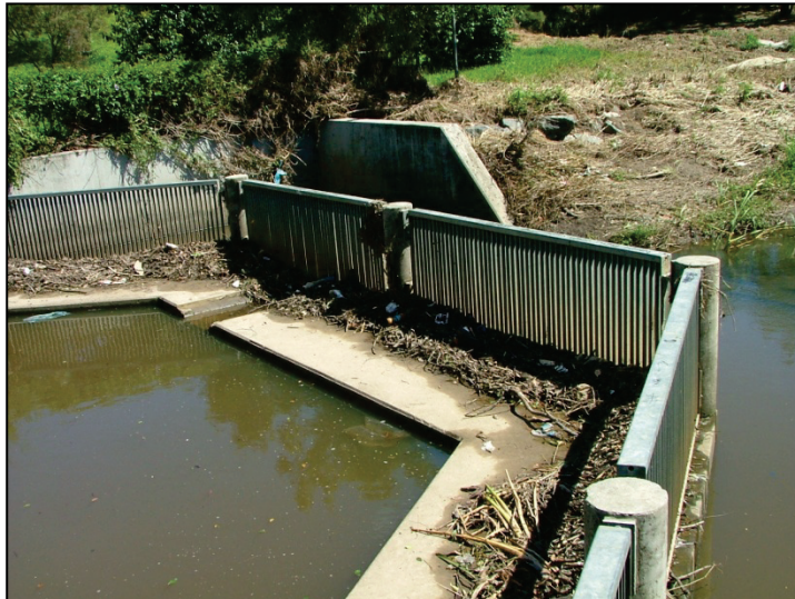
Figure 2.4 An open GPT consisting of a basin, a trashrack with vertical bars atop a weir located at Bedivere Street, Carindale on the outskirts of Brisbane (November, 2008).
