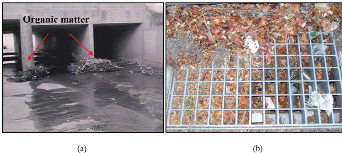
Figure 3.3 (a) A stormwater channel at Kingsgrove, 1954, (Image courtesy of The State Library of NSW) and (b) View of a stormwater drain fully blocked with organic matter at Graham Street in South Brisbane, 2008.
