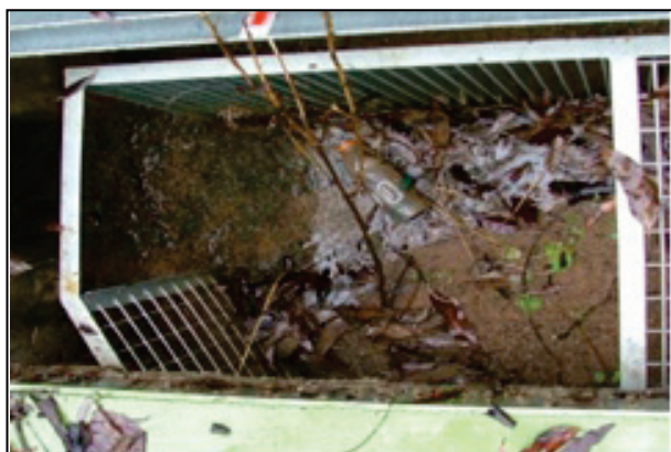
Figure 9.12 A snapshot of a field investigated GPT showing deposits of sediments which are similar to the pattern from the gross pollutant capture/retention experiments with partially buoyant spheres (See Figure 9.11). Note the blocked inlets in both cases.
