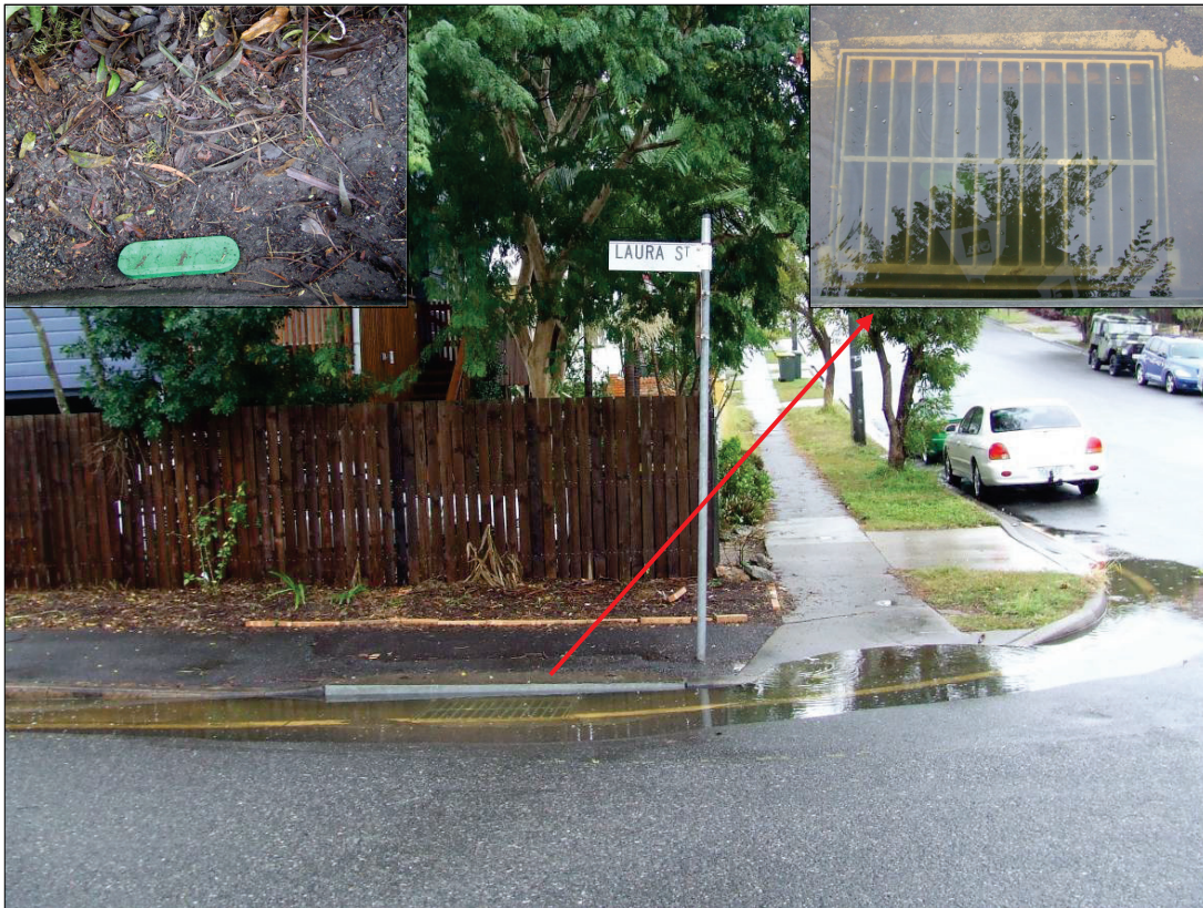
Figure 4.9 A view of the stormwater inlet drain (SWD No. 74 (See Tables 4.1 and 4.2) at the corner of Laura Street and Prospect Terrace, Highgate Hill) blocked with organic matter in a residential suburb of Brisbane. Inside the drain is shown on upper left and upper right is the top view.
