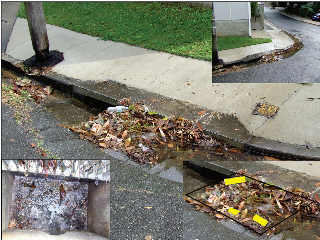
Figure 4.4 Storm water inlet drain in a residential area (West Street, Highgate Hill) of an inner suburb of Brisbane City clogged mainly with organic matter (small amounts of litter—plastic bottles and paper) just after a wet weather flow. Lower left is a view inside the drain (empty) and the top right shows the view of street and the drain location (June 2008). Lower right, the shaded area is used to map and estimate the gross pollutant contents (see SWD No. 75 in Tables 4.1 and 4.2).
