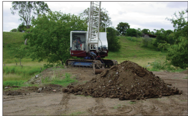
Figure 15. Photo of spoil pile after 50 autonomous cycles with the scale dragline in the background.
