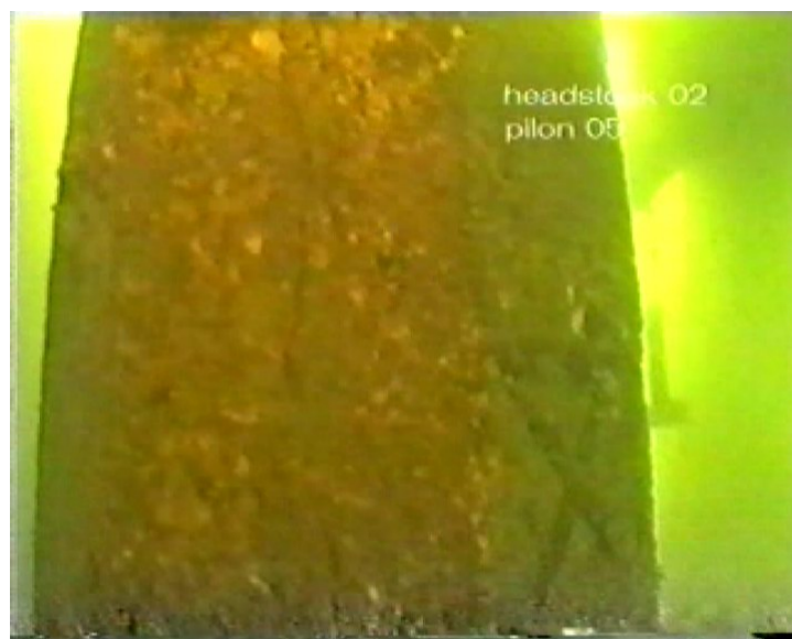
(vi). Underwater cracks in piles...contd..
