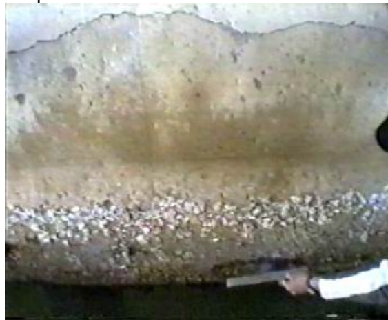
(i). Cracking near tops and soffits of the sides of a pilecap.
