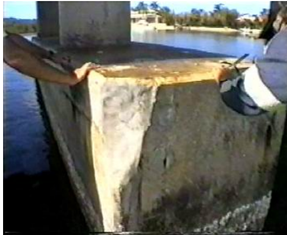
(iii). Cracking observed on the ends and corners.
