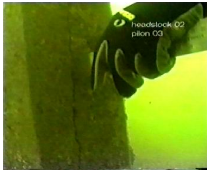
(ii). ASR observed in piles
