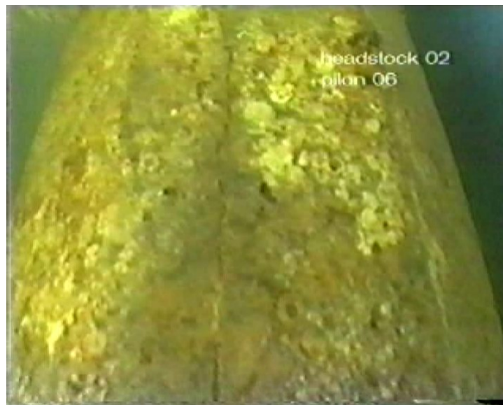
(iii). Underwater cracks in piles...contd..
