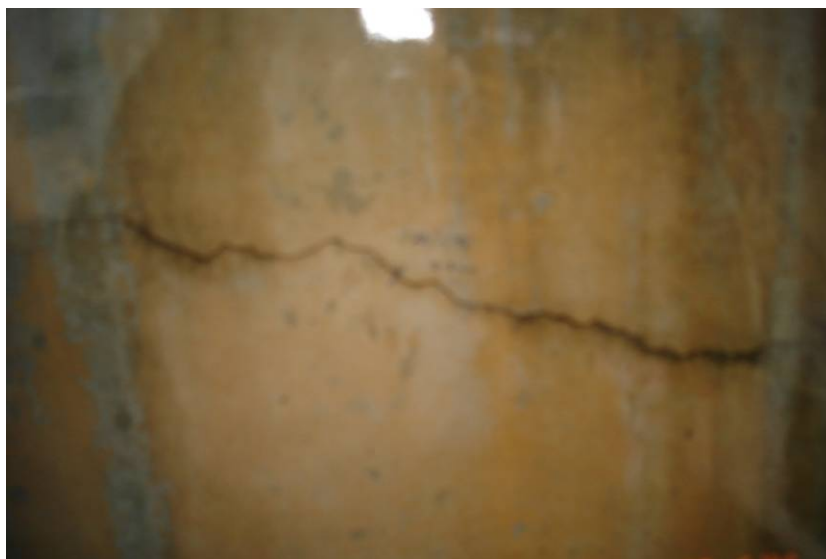
Photo 10a. Typical ASR cracking in bridge kerbs (a) Longitudinal cracking
