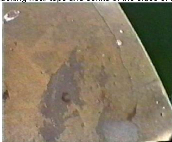
(ii). Cracking observed on top of the pilecaps.
