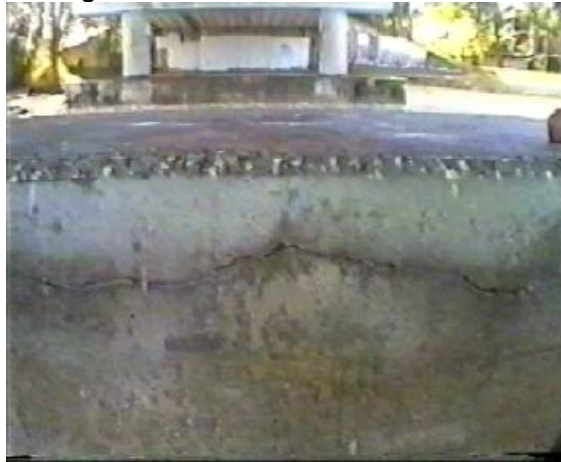
(iv). Cracking observed on the pilecap sides.
