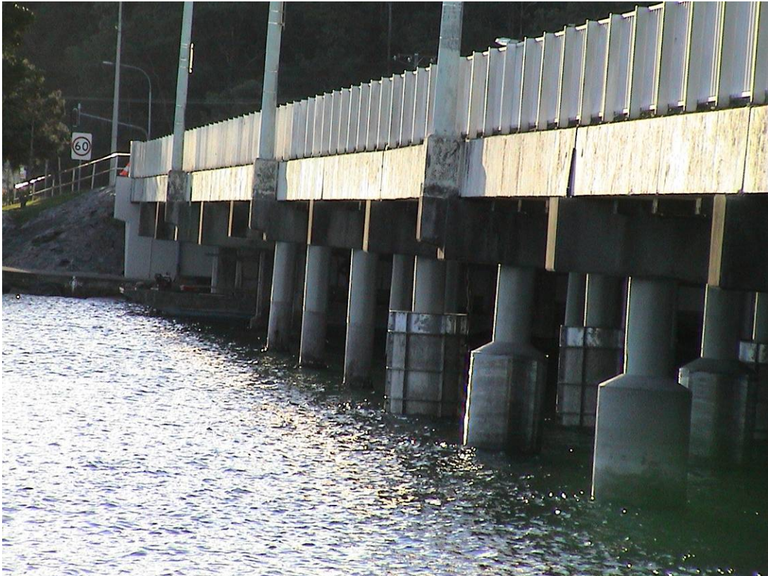
Photo 8. Typical appearance of Concrete encasements in bridges [Encasements constructed within 1 m of the headstock. The tops of the hollow spun piles wrapped with a carbon fiber system]
