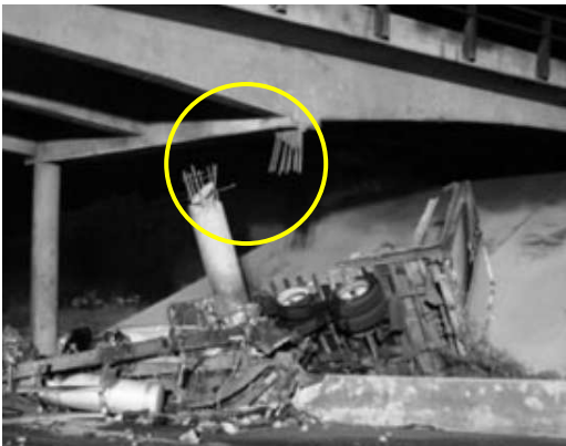
Figure 11: Damaged column under vehicle impact
