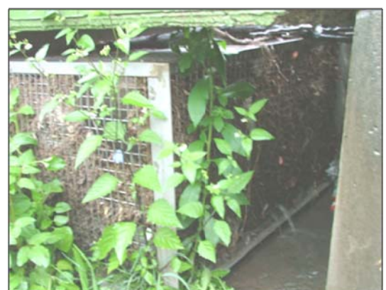
(c) Fully blocked screens.
