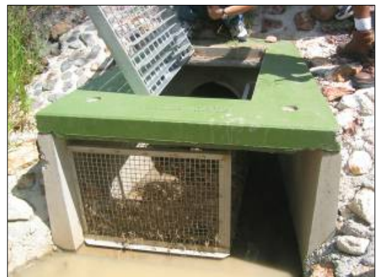
(b) Front view of a partially blocked screen with organic matter from incoming stormwater.
