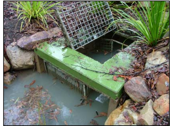
(a) High tide downstream causes flooding in the GPT LitterBank.
