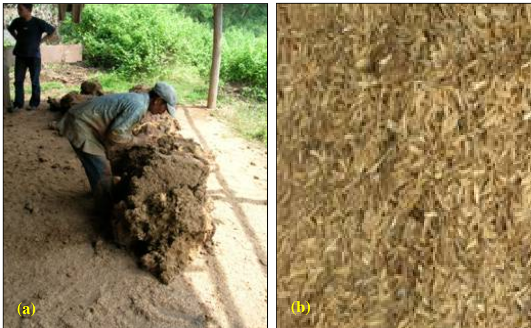
Figure 2.19 Process of mixing brick ingredients (a) Mixing clay paste and rice husk, (b) Rice husks
