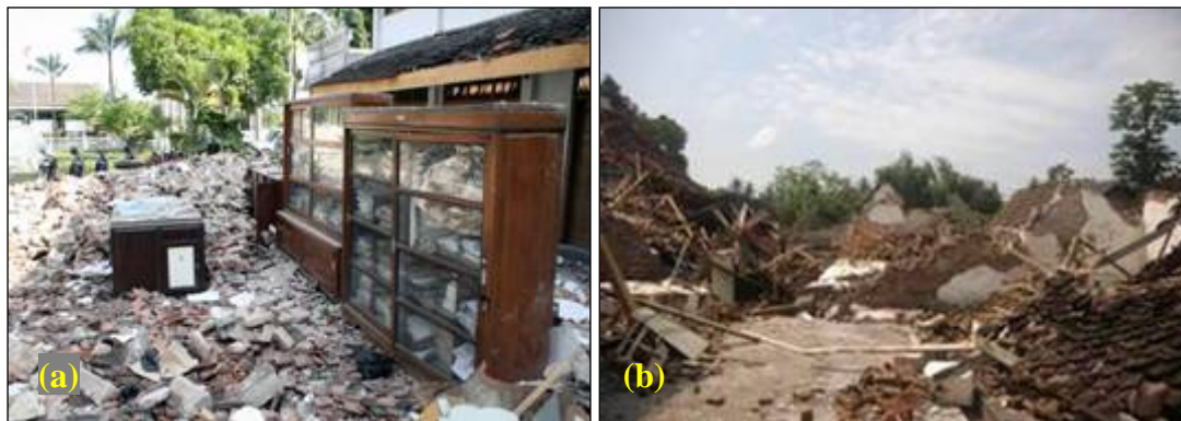
Figure 2.8 Damage on masonry houses during Nias Earthquake, March 2005 (a) Severe damage, (b) Total collapse
