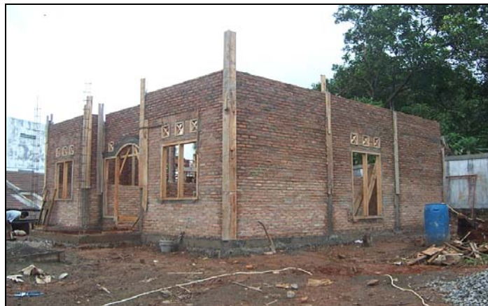
Figure 2.12 Masonry house without tie beam, during construction (Depok – 2005)
