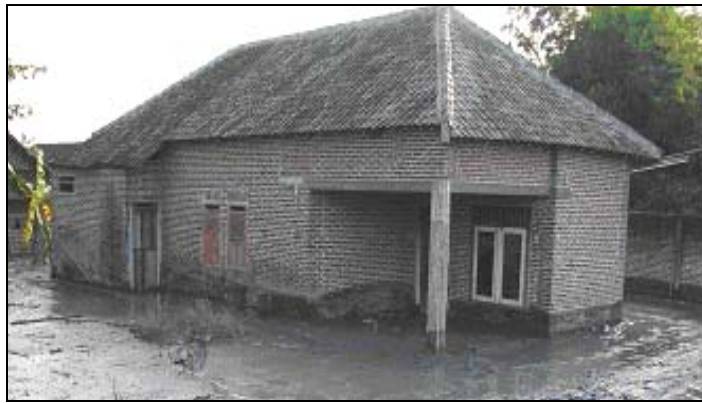
Figure 2.14 Masonry house without tie beam and column, viewed from corner direction (Porong - 2006)
