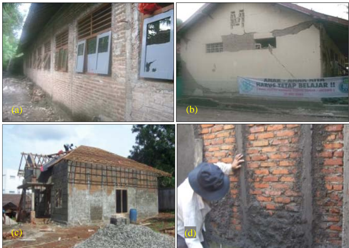
Figure 2.6 Brick wall for public elementary school building and houses (a) Without surface mortar, (b) Plastered with surface mortar (c) Plastered with comforted mortar, (d) Process on wall plastering
