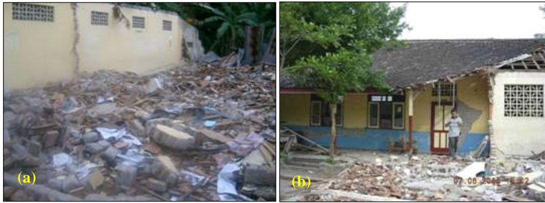
Figure 2.7 Damage on masonry houses during Yogya Earthquake, May 2006 (a) Severe damage, (b) Partial damage on mortared walls
