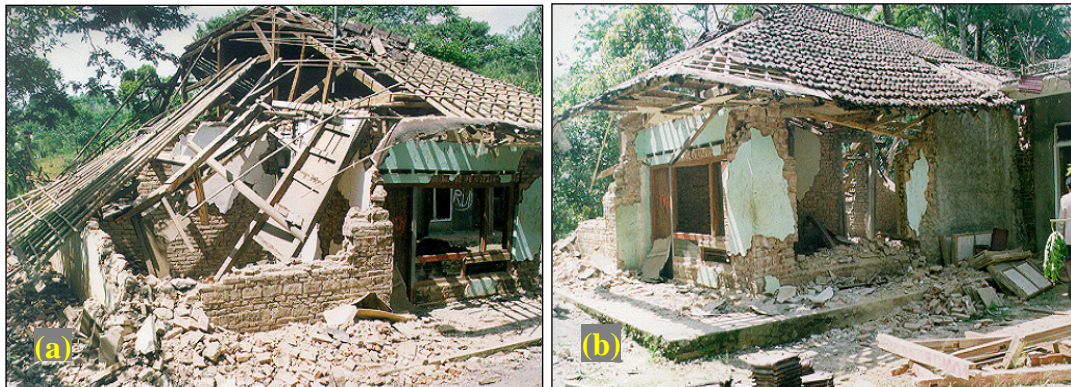
Figure 2.9 Damage on masonry houses during Majalengka Earthquake, April 2001 (a) Severe damage, (b) Partial damage
