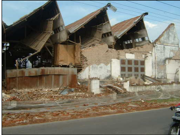
Figure 2.10 Collapse of the local industrial storage buildings during the earthquake
