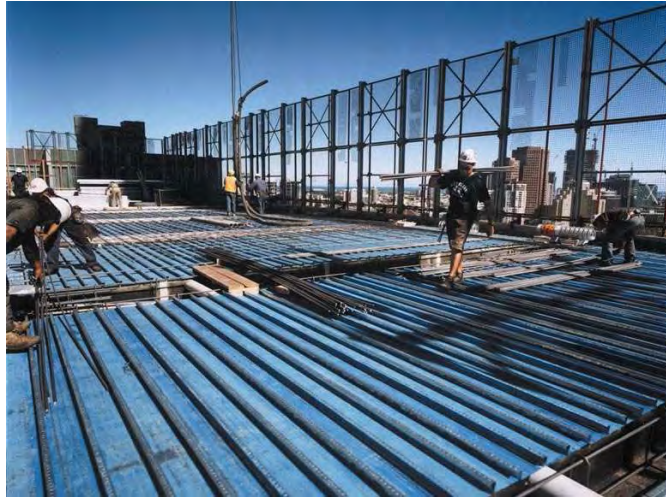
Figure 1-3: Composite floor in construction for a high rise office and residential complex in Melbourne
