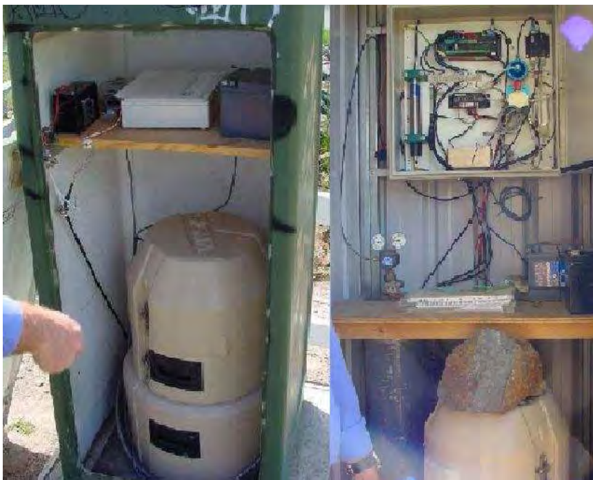
Figure 4.5 – Interior of automated monitoring stations
