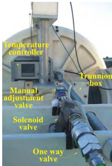
(a) Solenoid valve and temperature controller
