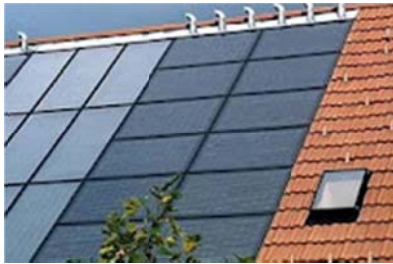
Figure 3: photovoltaic panels installed in a roof
