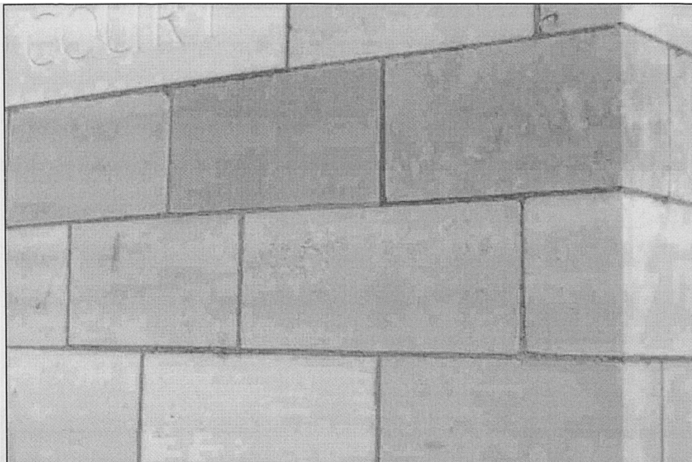
Plate 11 Rubbed ashlar wall, showing how the appearance is spoiled by errors of 2-3mm in location and joint width
