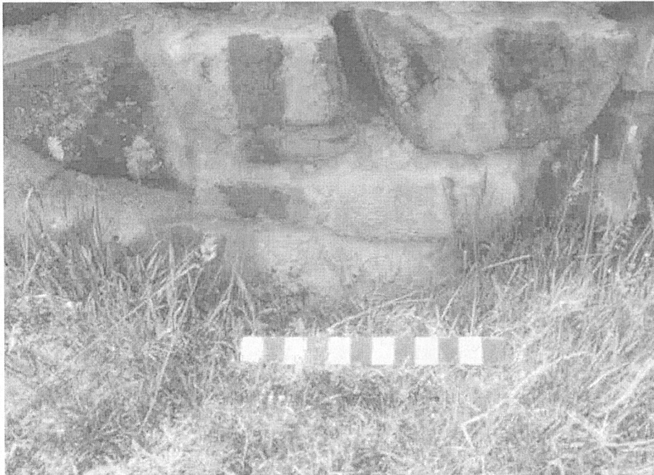
Plate 1 Lime from consolidation mortar leached out over facing stones, Peel Gap tower (1996)
