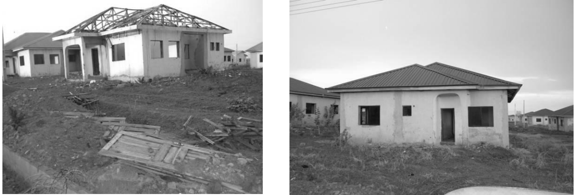
Fig 6: Views of the rehabilitative work depicting change in roof design and introduction of columns within walls. Source: Author's field work, 2011
