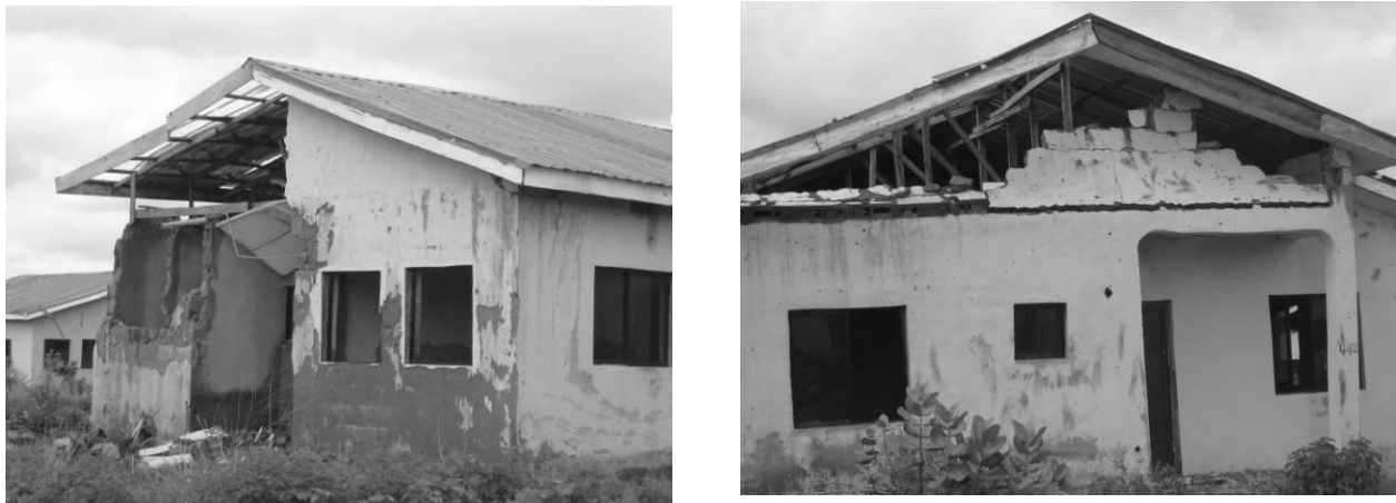
Fig 1: Two and three bedroom prototypes depicting widespread building material losses resulting in enormous construction waste. Source: Author, 2011
