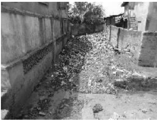
Plate 4: Refuse dumped inside drainage channels which hinders free flow of run-off Source: Field Survey, 2011
