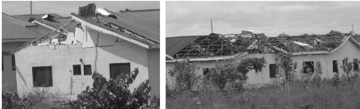
Fig 5: Views of the Talba housing estate depicting uniform pattern of material waste along the gable end owing to flawed roof design and poor building orientation. Source: Author's field work, 2011
