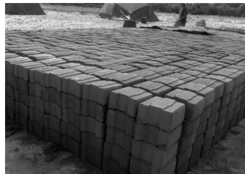
Pic 2: The Hydraform blocks ready for the first building. Source: Malaika Kids UK website.
