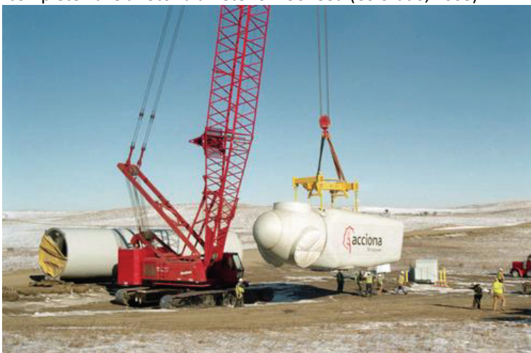
4b. Lifting the 163,000 lb. nacelle and rotor hub for a 1.5 MW turbine at Tatanka Wind Energy (North Dakota, 2007).
