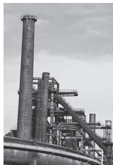
Figure 1 Effect of atmospheric corrosion
