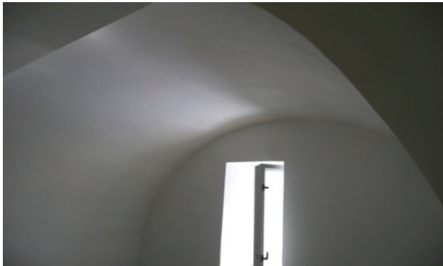
Figure 17 A view of interior arch after application of thermal insulating polyurethane mortar for plastering and after finishing (pargeting and painting)
