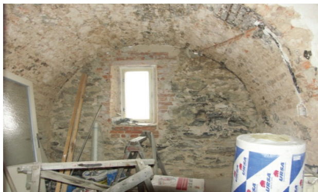
Figure 16 A view of interior arch and masonry without original plaster inside the building
