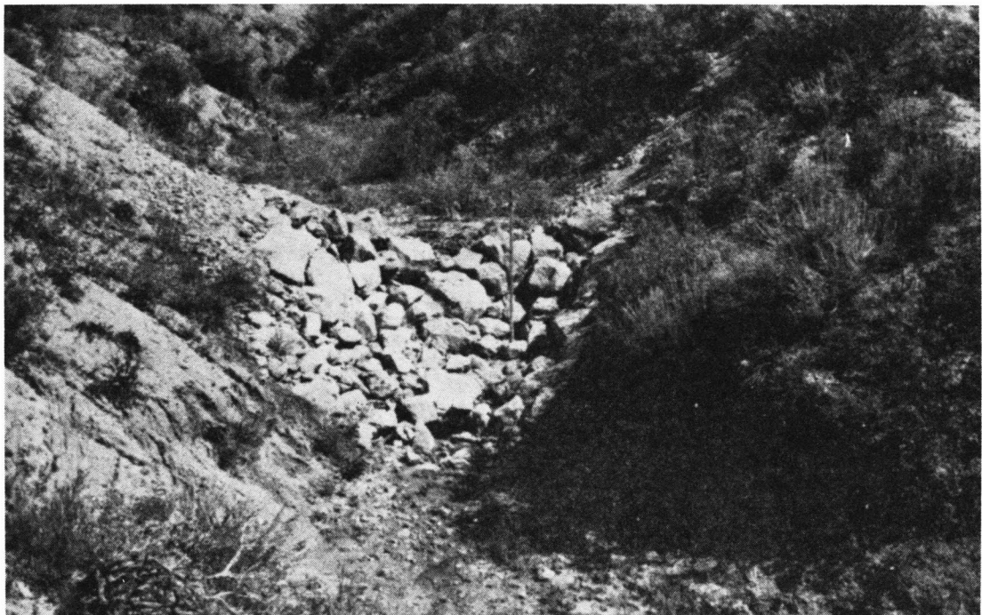
Figure 39. A rock-fill check dam. (Heede 1977)
