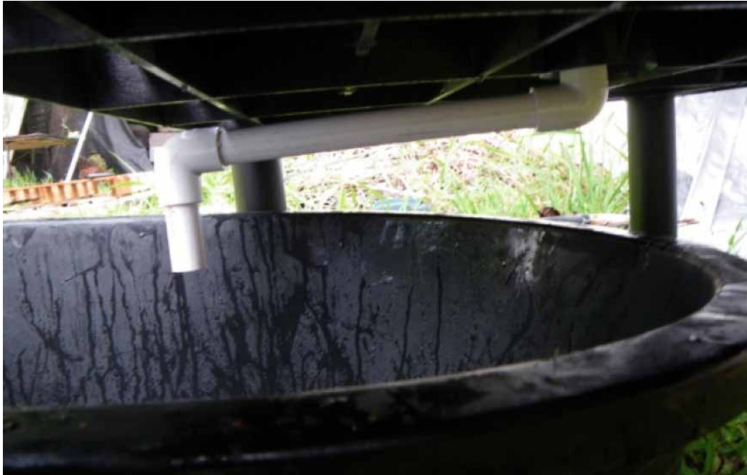
16. The drain assembly on the underside of the grow-bed. Note the two sequential 90° elbow fittings, which help start and stop the siphon and direct the flow of water back to the rearing tank beneath the grow-bed.
