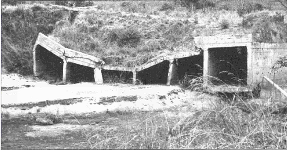
A collapsed bridge in Tanzania, now under repair
