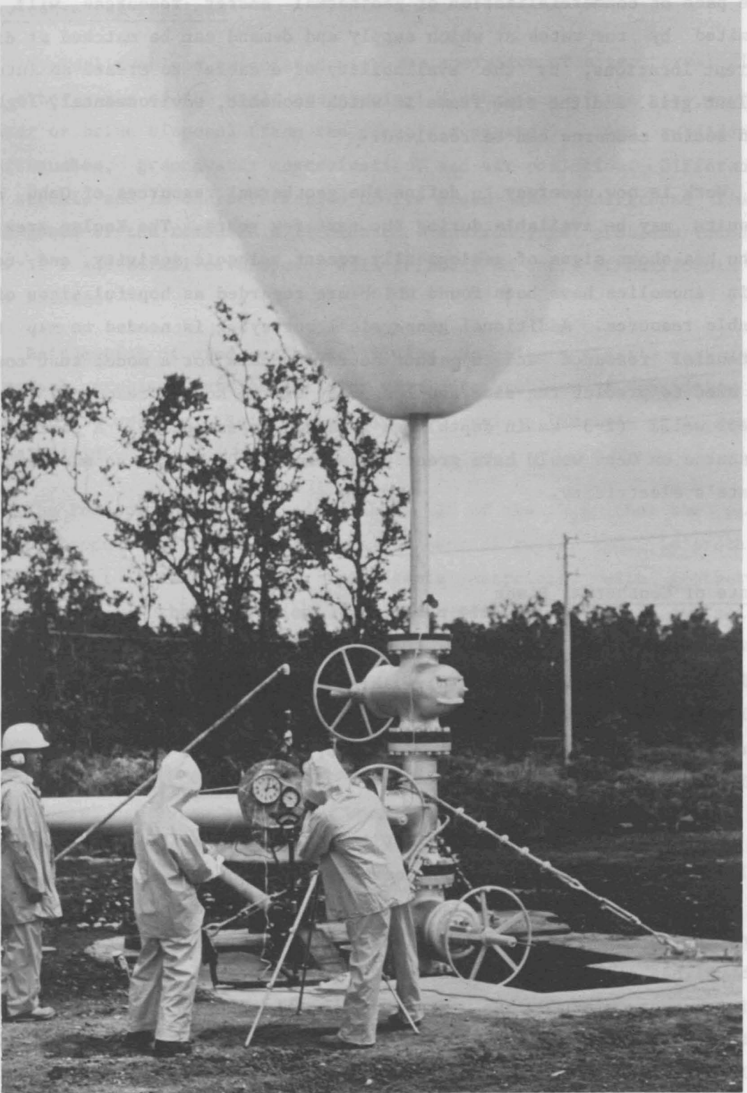
The HGP-A geothermal well on the Island of Hawaii.
