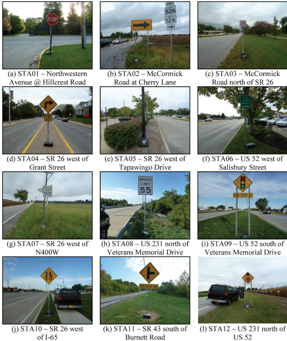
Figure 6.3 Bluetooth monitoring station installations.
