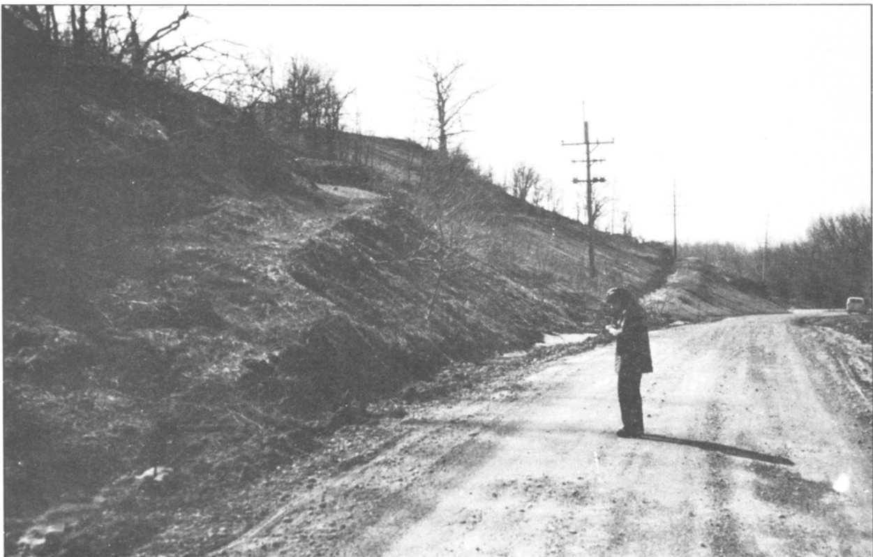
Figure 9 This slope (along the same road shown in figs. 7 and 8) has been benching in an attempt to stabilize it.
