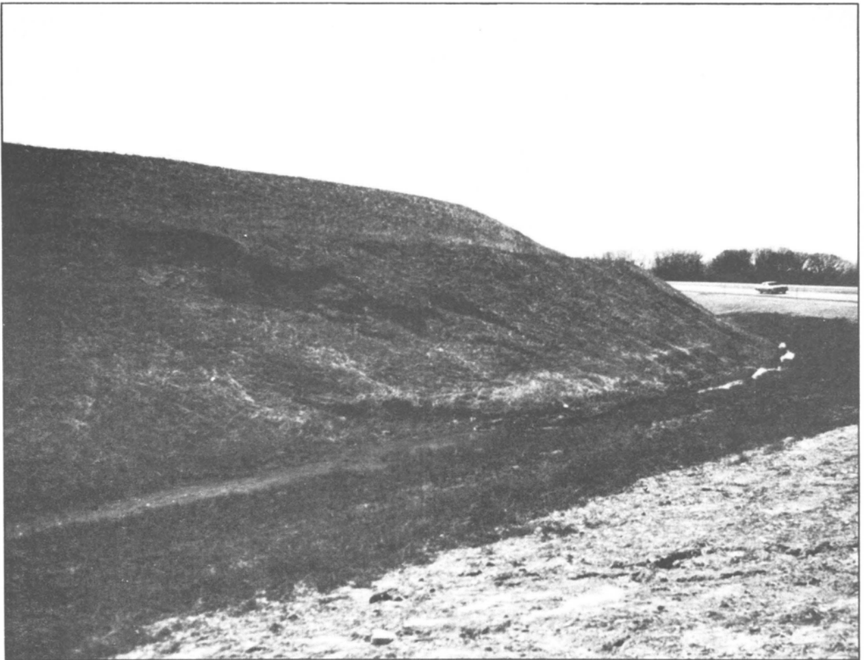
Figure 22 Shallow landslides ("skin" slides) occasionally develop along newly constructed highways where the uppermost layer of saturated soils turns into a viscous liquid and flows downslope.
