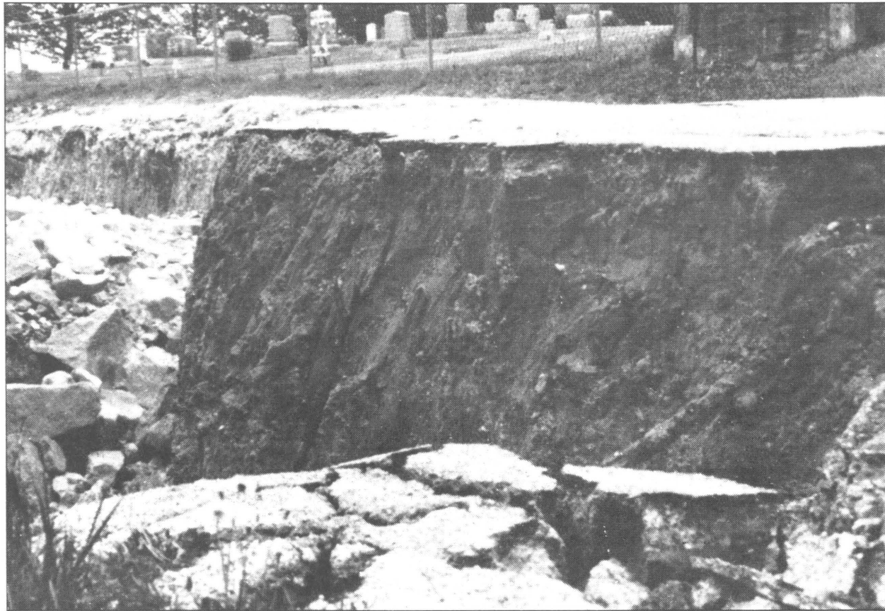
Figure 25 A close-up view (from the opposite direction) of the slide's main scarp. Blocks of asphalt roadway appear in the foreground. The crushed rock in the background, added to stabilize the slide, overloaded the uppermost slump unit and contributed to additional sliding. (Photo: S. C. Bradford, ISGS)
