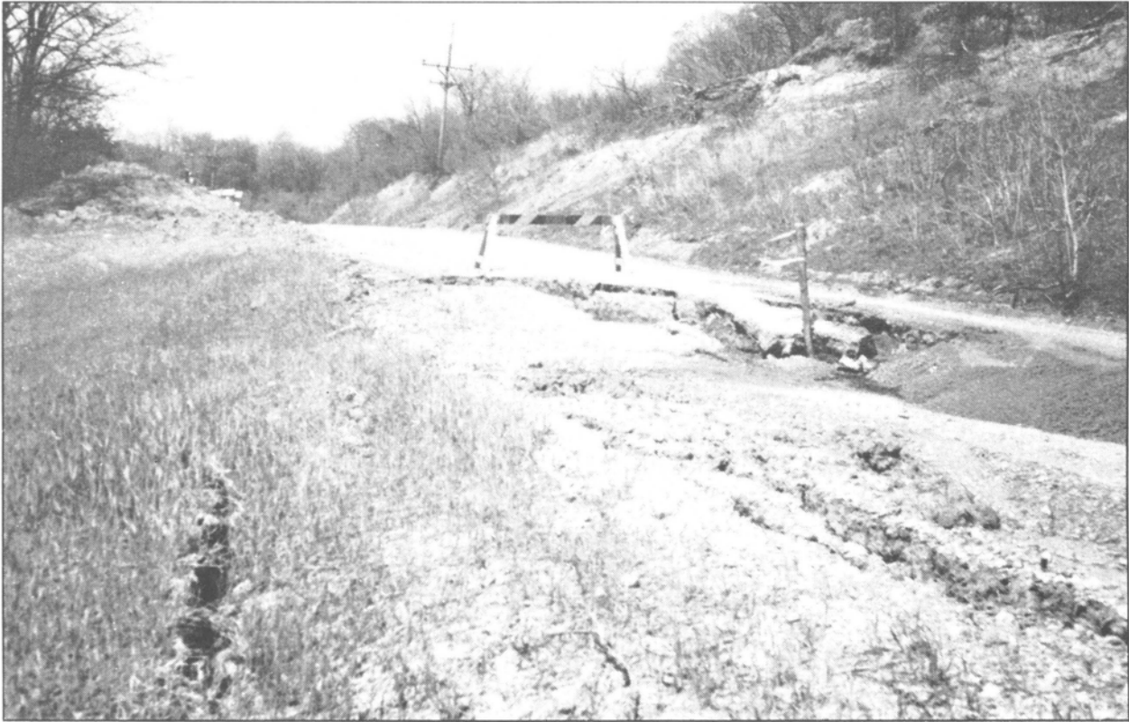
Figure 8 Road damage from additional slumping that had taken place by the time the authors revisited the same site 2½ weeks later. This photograph was taken from a spot behind the van (fig. 7). Slumping has also occurred on the hillside above the road.
