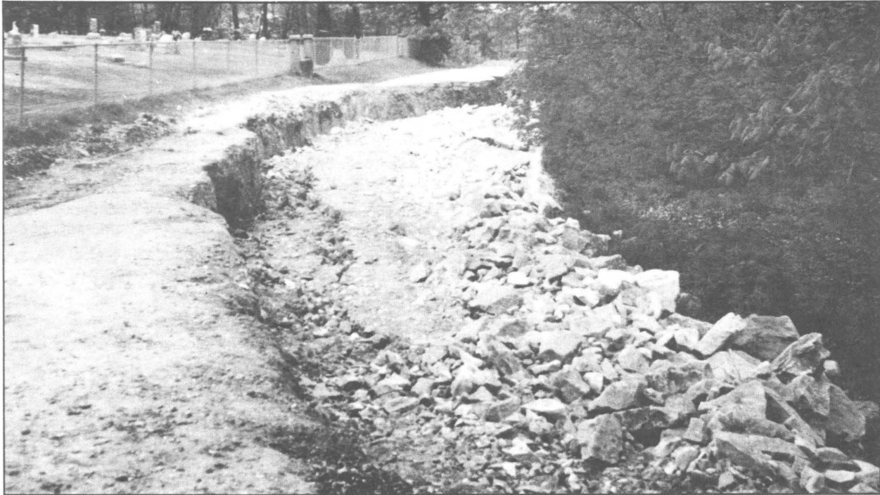
Figure 24 This earth slump in western Illinois was aggravated when a load of stone was placed on the uppermost slump unit to fill the area. Subsequent movement caused additional damage to the road.
