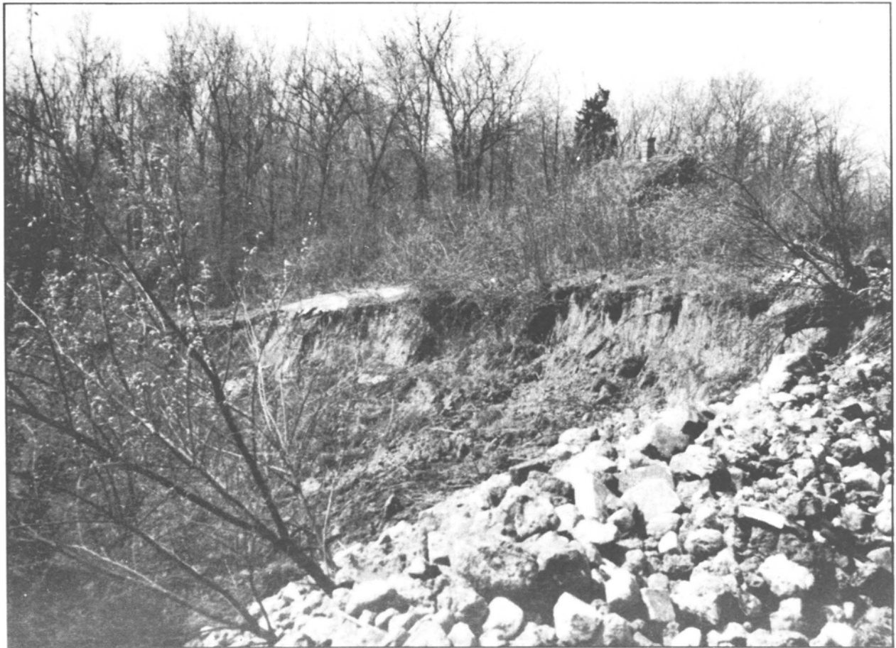
Figure 23 Crown and main scarp of a large earth slump on bedrock in bluffs west of the Illinois River. Note load of stone dumped on the main scarp along the crown in foreground. The trees were probably bent by the stone.
