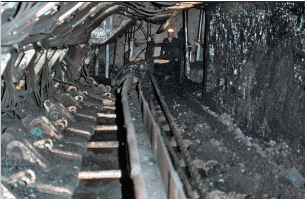
Figure 97 Old Ben Coal Corporation, mine and location unknown. The roof shields support the roof as the cutting drum mines the coal to the right. The longwall unit then advances to the right after one pass of the drum shearer. The roof behind the unit is allowed to collapse as the unit moves forward.
