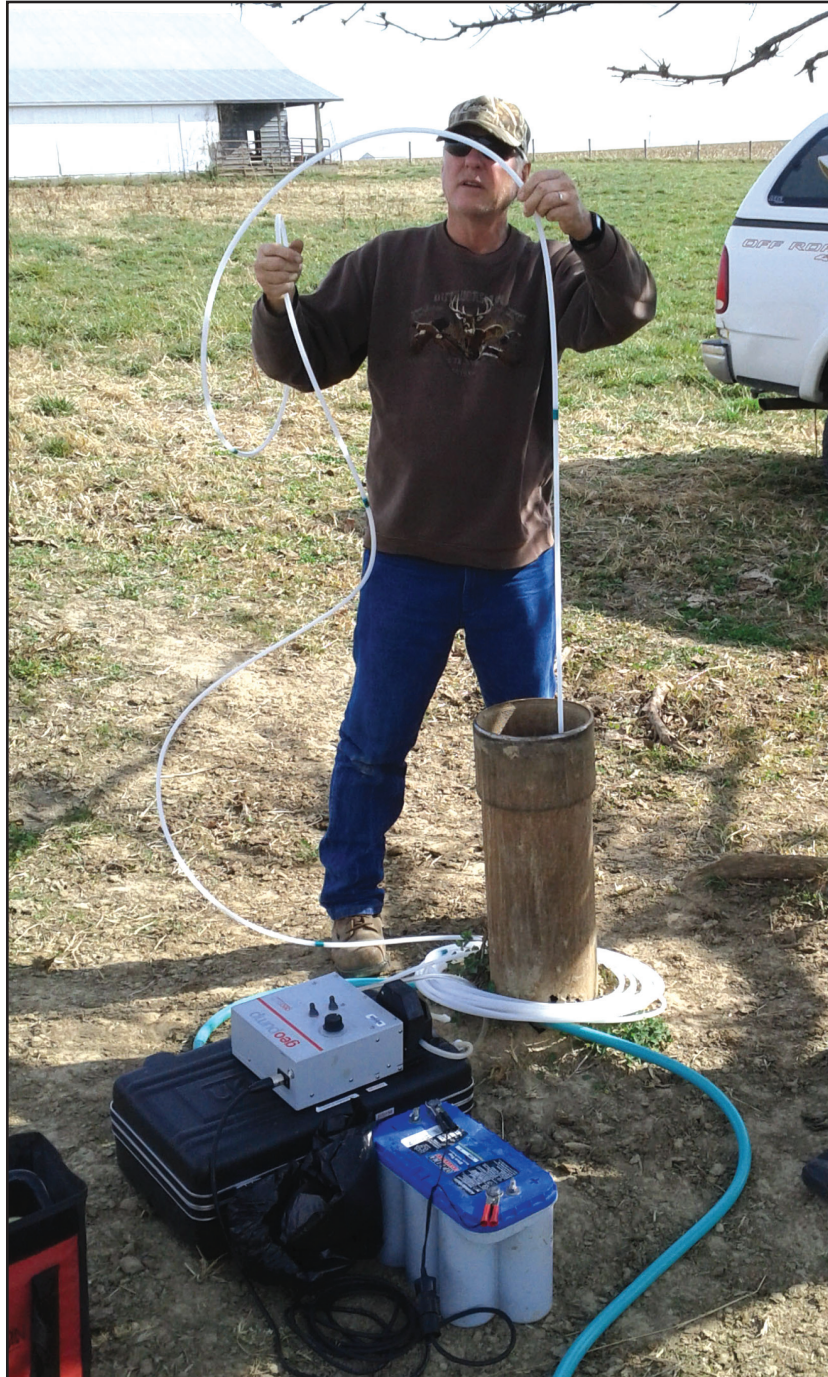
Figure 5 Private water supply well without active pump.
