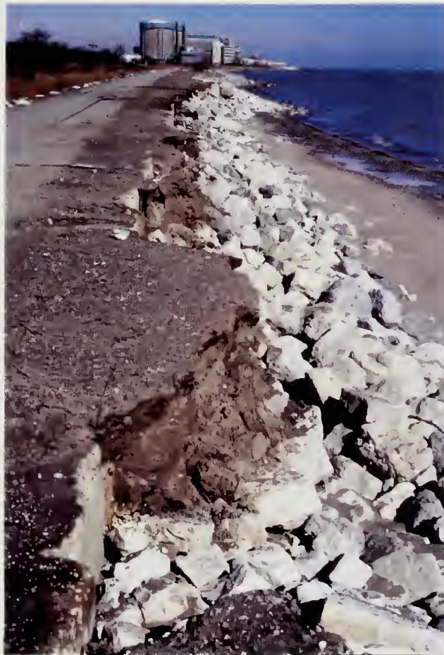
Figure 3-22 Photograph showing the south end of the IBSP/SU beach-nourishment site. A precipitous drop-off exists between road level and the adjacent riprap and beach. For scale, the concrete cubes in the foreground along the east side of the access road measure 3 ft by 4 ft by 4 ft. View is to the north with the Zion Nuclear Power Plant in the background (photo date February 25, 1997).
