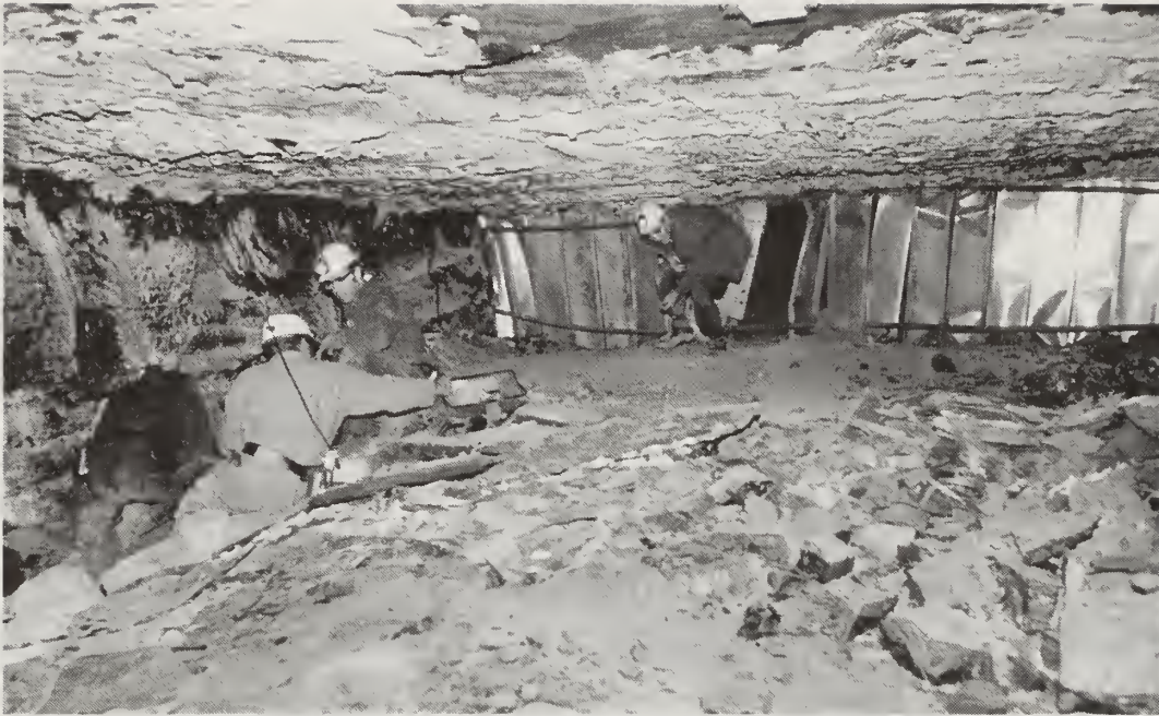
Figure 28 Floor squeeze in an underground mine in Illinois.
