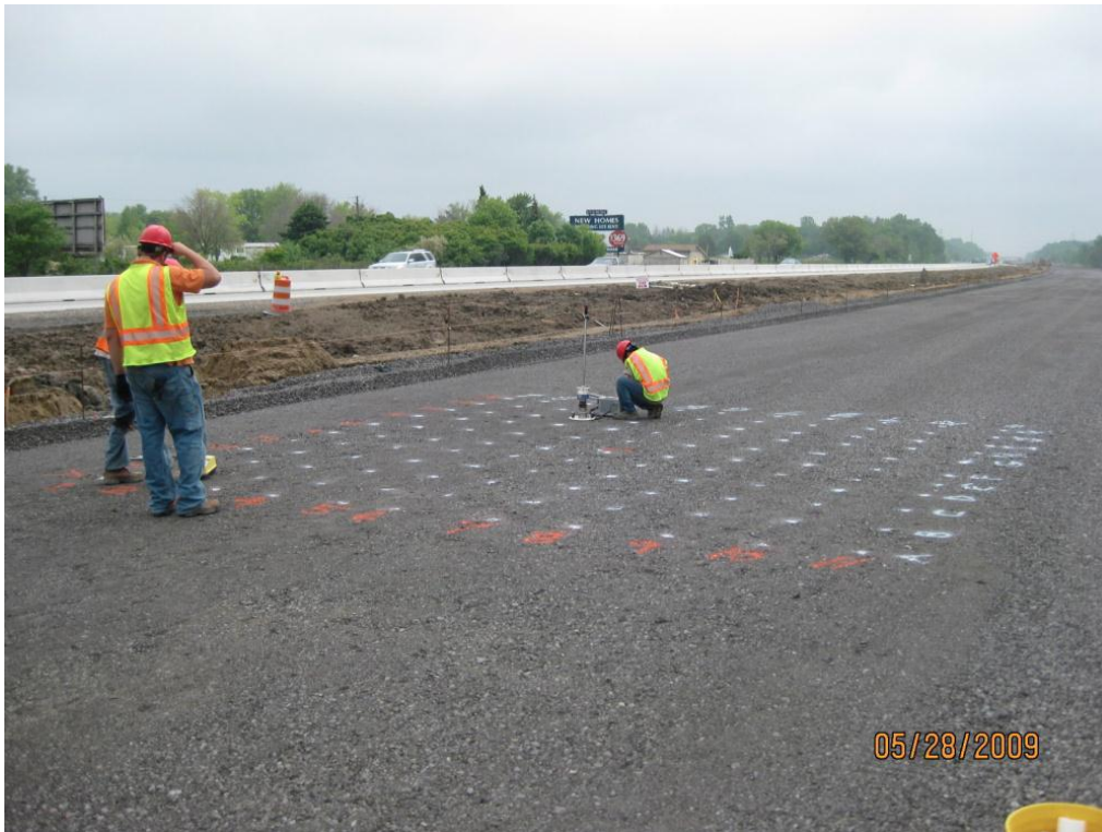
Figure 3: DCP test being carried out on an OGDC layer on test bed 1b (34)
