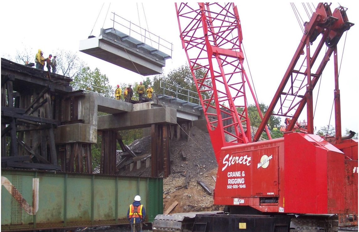
Figure 5.2. Partial replacement of a timber trestle railroad bridge in the Midwest of U.S.
