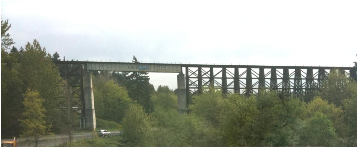
Figure 4.3. Timber trestle bridge over passing a highway with the help of a DPG by Seattle, Washington State (currently not open to traffic).
