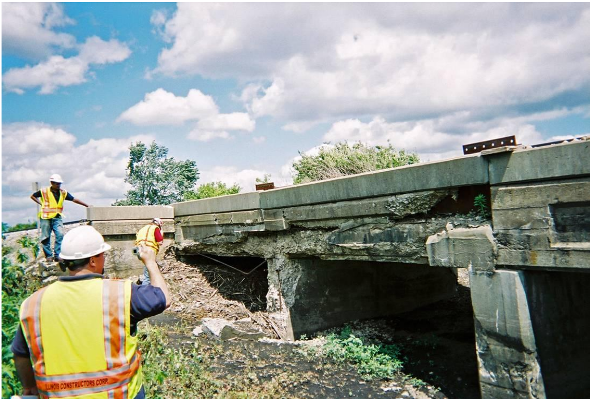
Figure 4.2. Railroad bridge deck slabs over hundred years old replaced by the CN and tested to estimate their ultimate load capacity.
