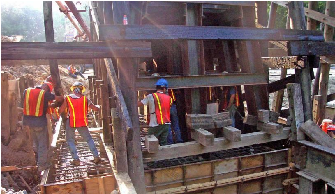
Figure 5.7. Concrete collar installation in a maintenance intervention for a railroad bridge partial replacement (Class I railroad).
