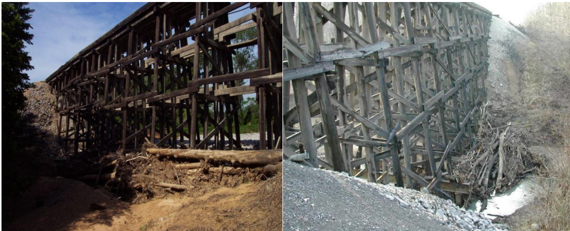
Figure 4.12. Debris accumulation on tall timber trestles after seasonal rains.
