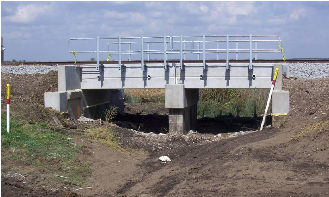
Figure 5.1. Maintenance results in a 100 year old railroad bridge superstructure replacement, while keeping the substructure, which was found in good condition.
