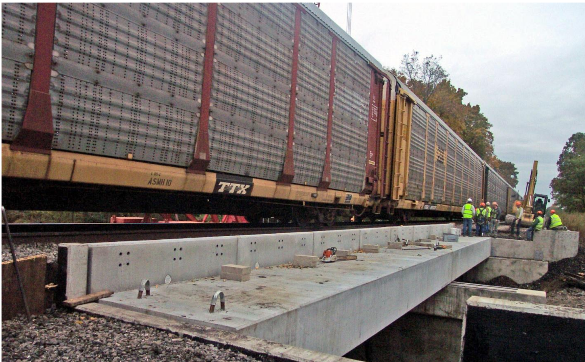
Figure 5.8. Complete railroad bridge replacement in a main line with more than 26 trains/day (no work windows allowed).
