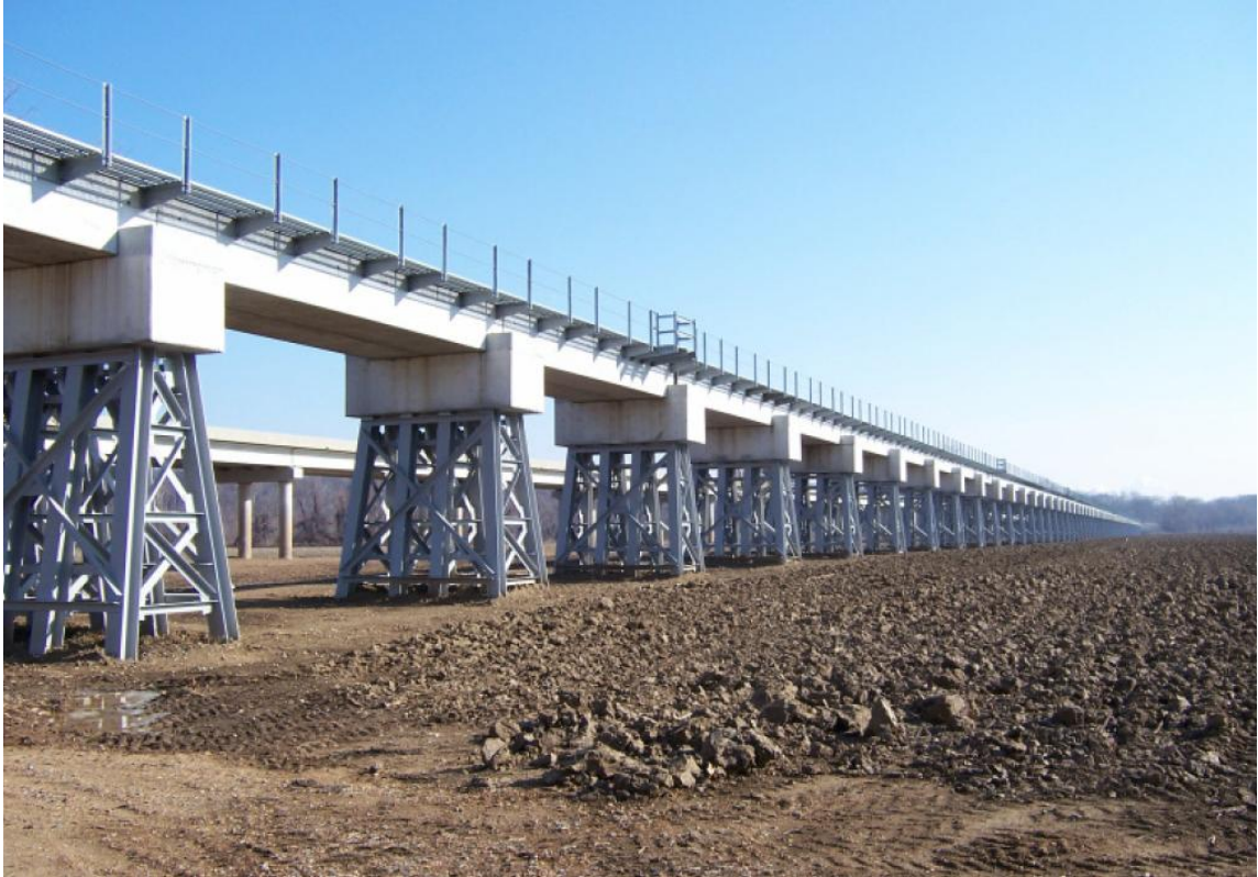
Figure 4.11. New Class I railroad bridge viaduct replacing a railroad timber trestle in Kentucky.
