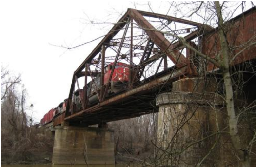
Figure 6.7. Class I railroad bridge with a main truss span and two plate through approaching spans.
